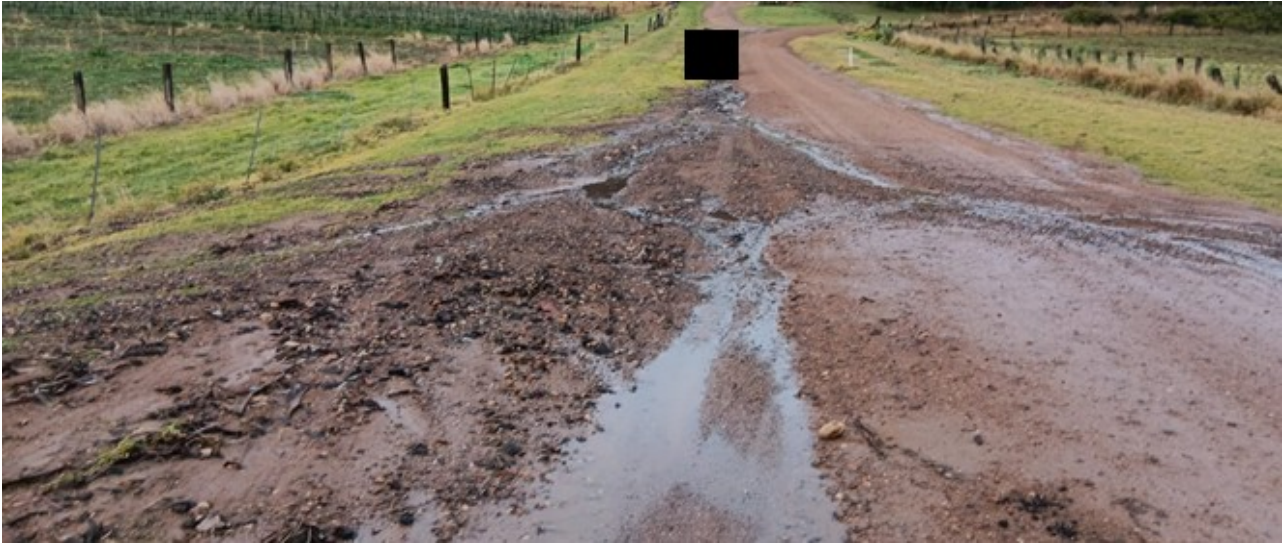
Figure: Erosion and sediment loss due to drainage constraints near proposed passing bay location on Pokolbin Mountains Road, not identified or assessed in the EIS (photo June 2025) [edited for privacy]
