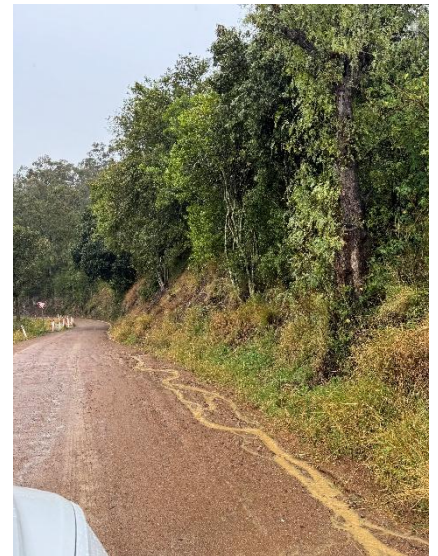
Image 5 Pokolbin Mountains Road - 1 day after grading with moderate rainfall
