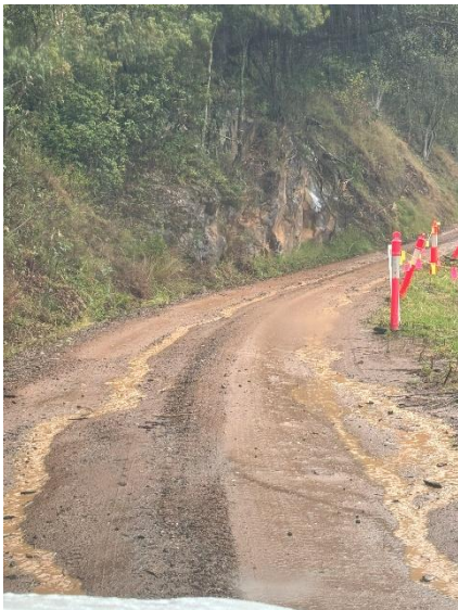
Image 3 Pokolbin Mountains Road water guttering due to lack of drainage
