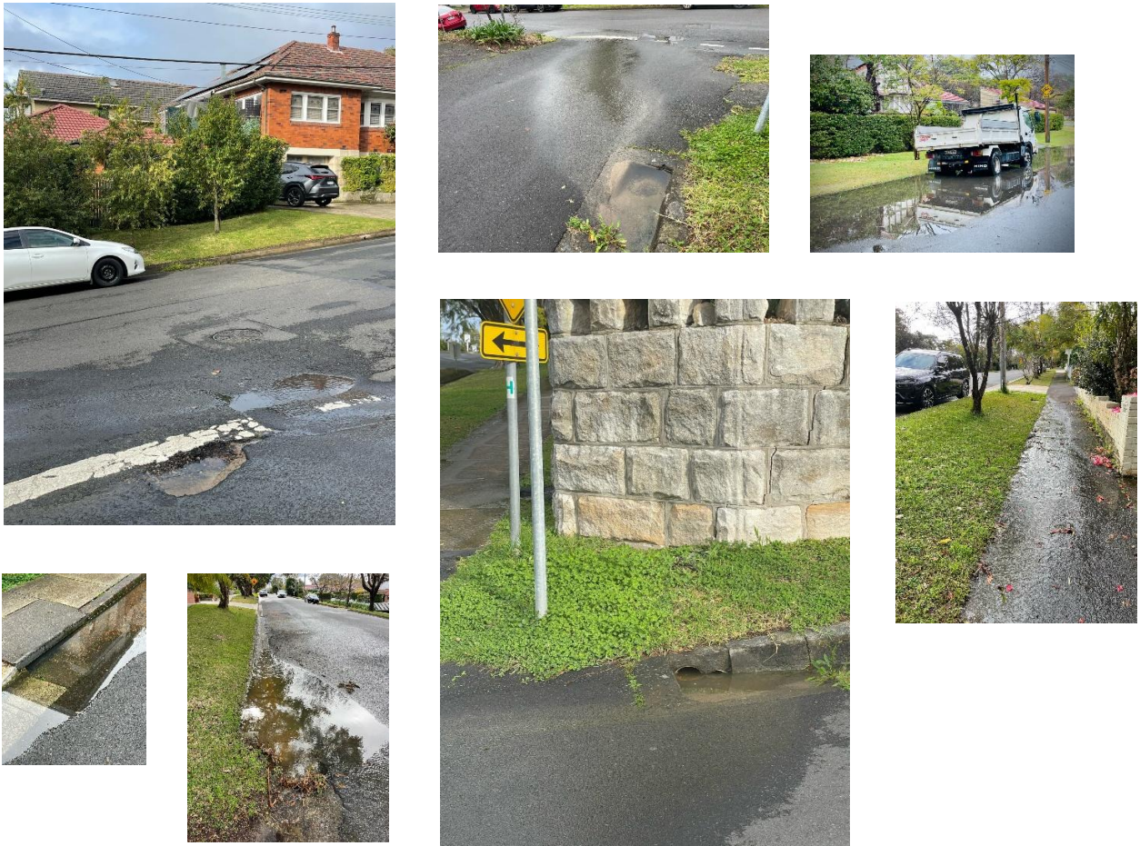
Figure 8. Overflowing stormwater drains are a common sight in the location, including immediately across from the proposed site, reflecting the ageing infrastructure, that is not able to cope with high density, including the 5,500% in dwelling density on the site in question. Other infrastructure not able to cope include roads, parking, and the ageing North Shore state rail line, which today experiences substantial delays and low frequency of trains compared to the newly built Metro system servicing newer suburbs across Sydney.
