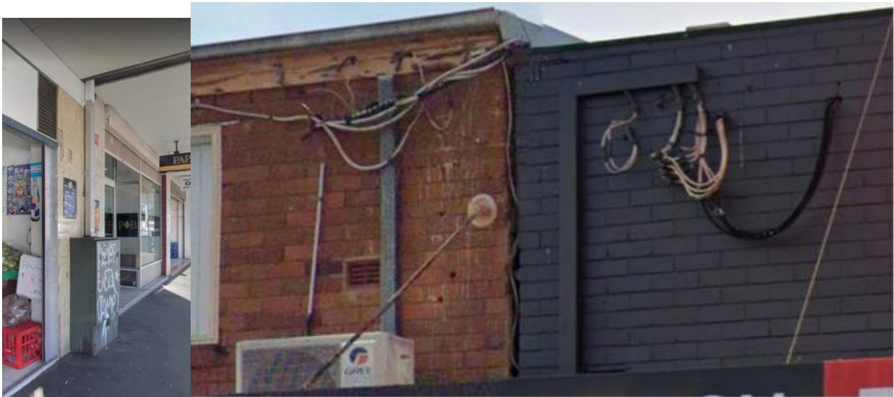
Example of 'awning' overhead power lines coming from a low voltage pillar on the road verge rising to through a duct and then through or above the awnings to the customer connection points for the premises. Source: Google Maps Street View.
