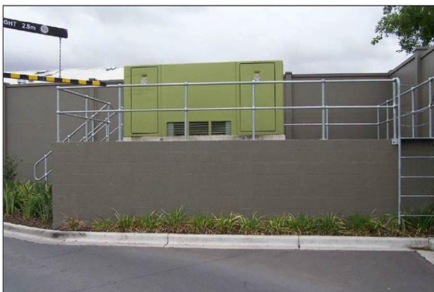
Figure 51 - Example substation raised above 1:100 flood level
