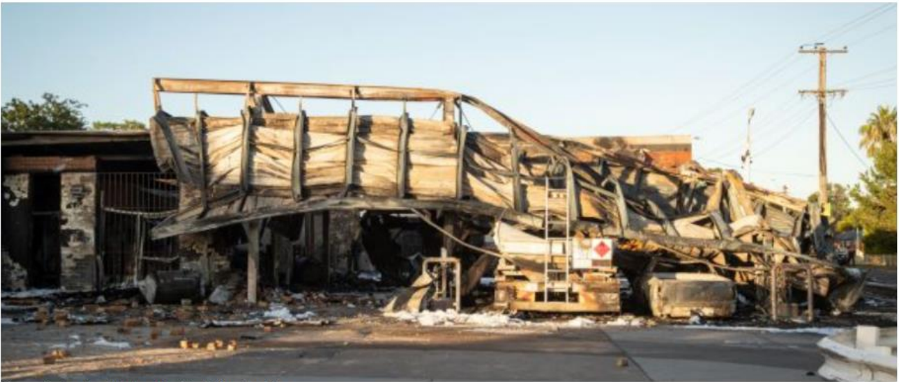
Figure 4: Service Station Facility Following Fire
