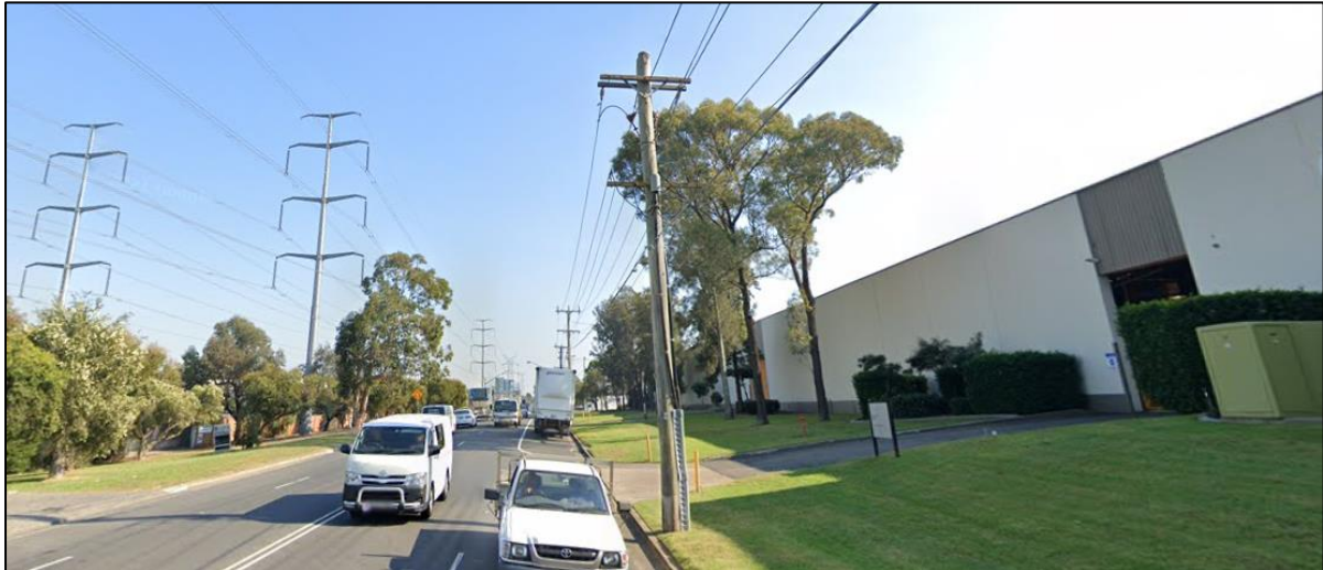
Transmission, high voltage and low voltage overhead power lines in Long Street Smithfield. There are also high voltage underground cables coming from the pole going to the padmount substation. Source: Google Maps Street View.
