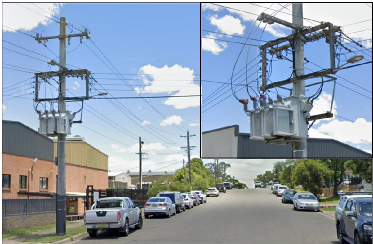
Pole mounted substation in Wellington Street Riverstone. Source: Google Maps Street View.
