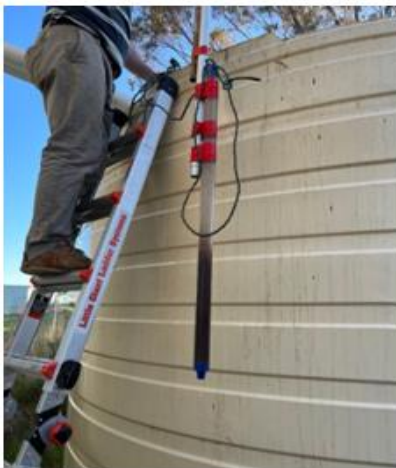
Tank approximately 10-15 years old galvanised shed and plastic pipes. Never cleaned.
