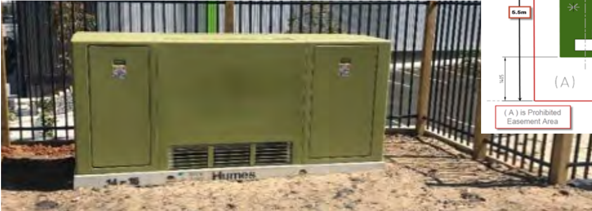
Example of a padmount substation
