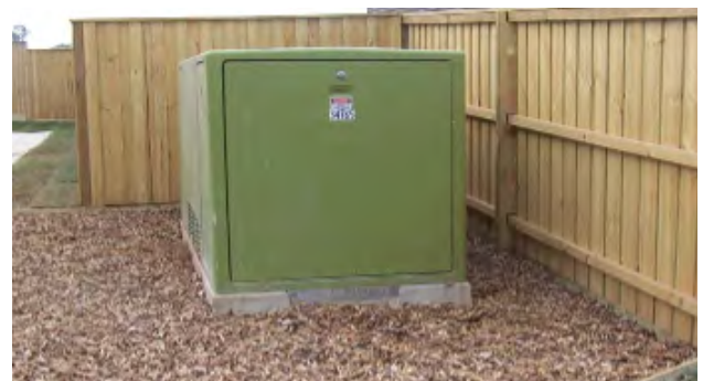
Correctly maintained padmount surrounding area
