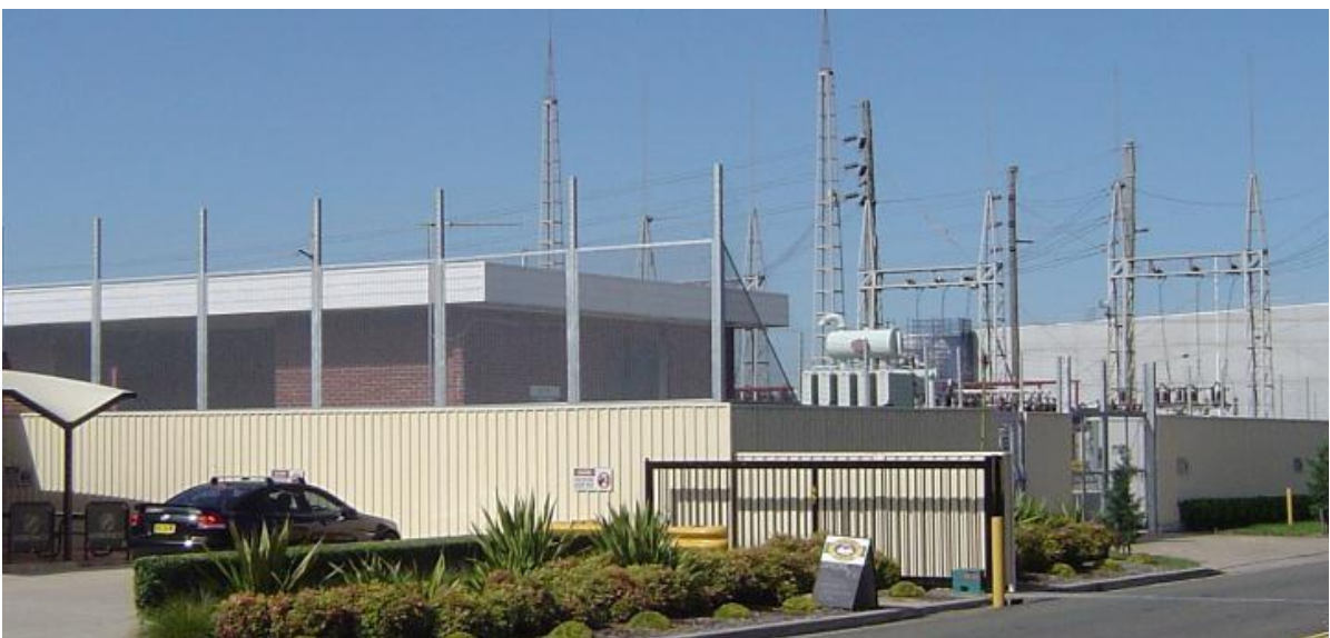
Endeavour Energy's Seven Hills Zone Substation is an 'outdoor' design. Note height of fencing due to adjacent 'climb point' created by the seating and awning.
