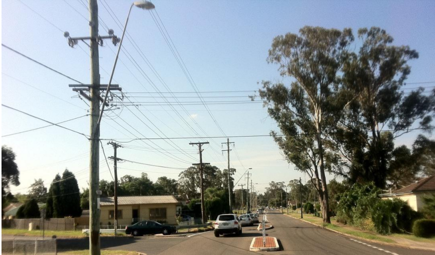
Overhead powerlines with high voltage, low voltage and service connections at different levels on the poles. This example is in Marayong NSW part of Endeavour Energy's franchise / network area. Source: Google Maps Street View.
