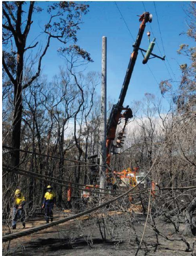
Endeavour Energy crews replacing a burnt timber pole with a concrete pole after the September 2013 bush fire at Winmalee NSW. Source: Everyday Endeavours, Staff Newspaper November 2013
