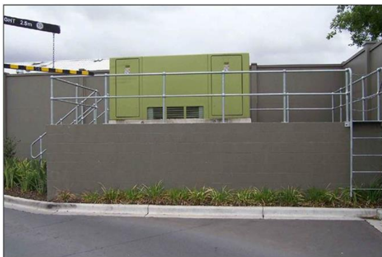
Figure 51 - Example substation raised above 1:100 flood level
