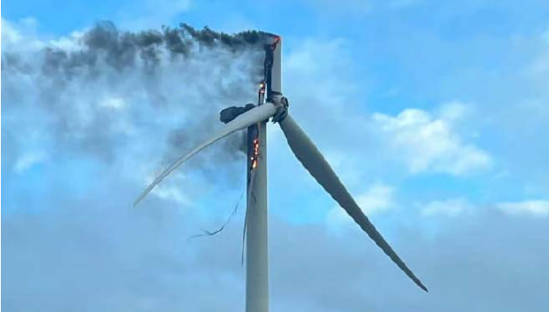
Goulburn Wind Turbine Fire January 2023
