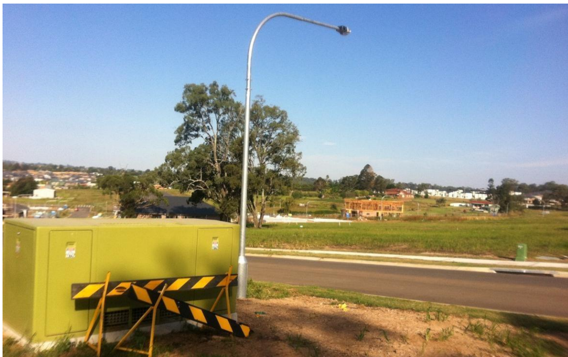
Padmount substations are converters of electricity, reducing the high voltages for street lighting and to the end user whilst low voltage pillar boxes are distribution junction points. These structures also mean underground cables are nearby. Digging activities and planting of trees or shrubs should not occur near them.
