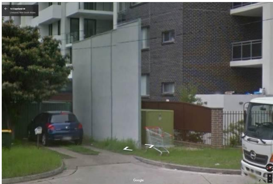
Fire wall constructed for padmount substation at 18 Copeland Street Liverpool. Source: Google Maps Street View.
