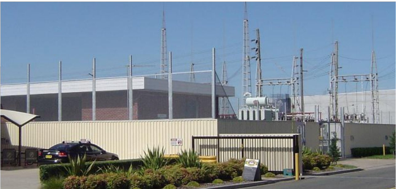
Endeavour Energy's Seven Hills Zone Substation is an 'outdoor' design. Note height of fencing due to adjacent 'climb point' created by the seating and awning.
