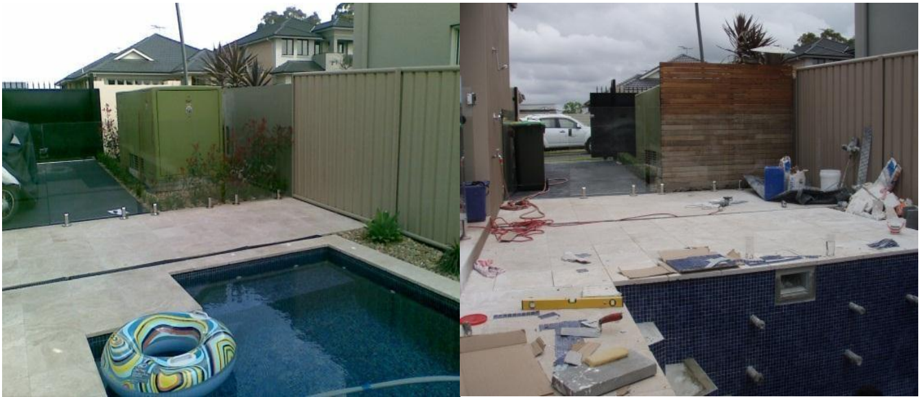
Before and After. This swimming pool in Endeavour Energy's network area at Middleton Grange NSW had to be modified to comply with the restriction for the padmount substation on the use of land in relation to swimming pools.
