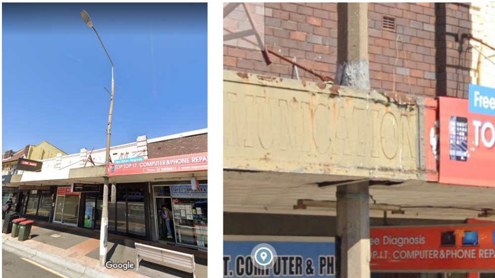
The street awning is inappropriately constructed around the streetlight column. Source: Google Maps Street View.
