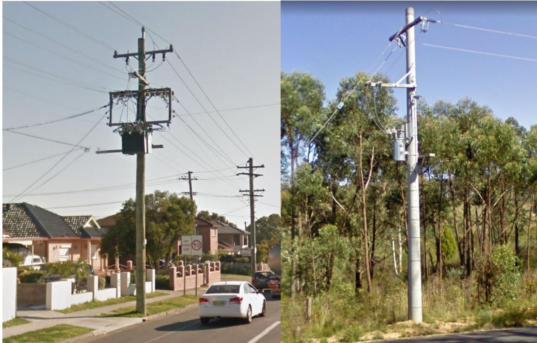
Pole mounted substation no. 914 in Blaxcell Street, Guildford NSW has 79 customer connection points servicing 119 premises in an urban context which is at the upper end of the number of premises able to be serviced. In contrast pole mounted substation no. 26132 in Baaners Lane Little Hartley NSW in a non-urban context only services a single rural property. Source: Google Maps Street View.
