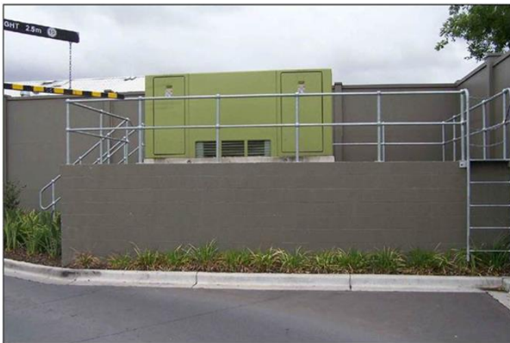
Figure 51 - Example substation raised above 1:100 flood level
