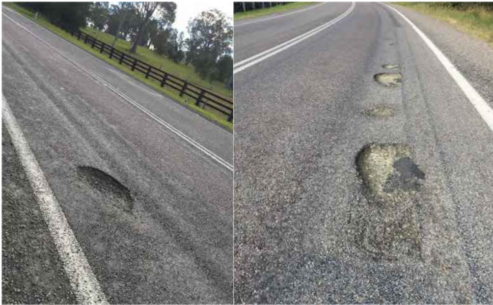
Tocal Road, pavement failure
