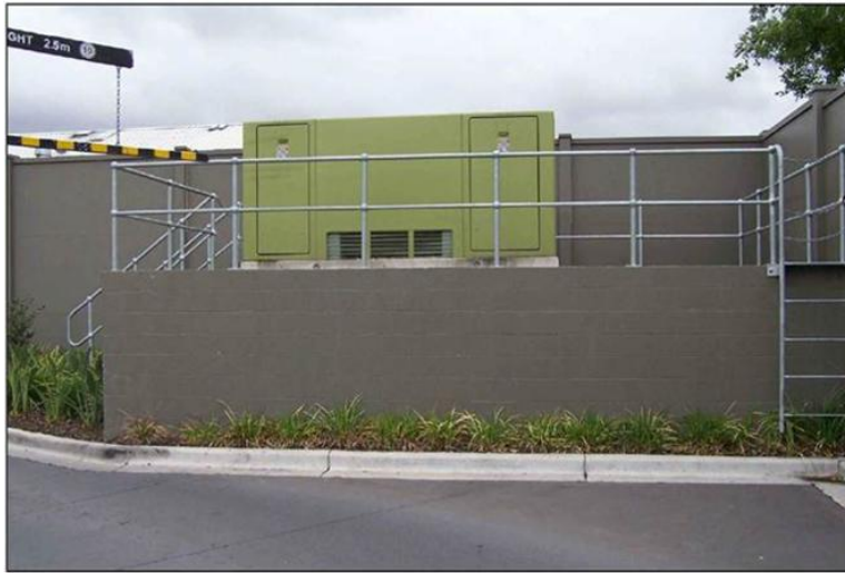
Figure 51 - Example substation raised above 1:100 flood level
