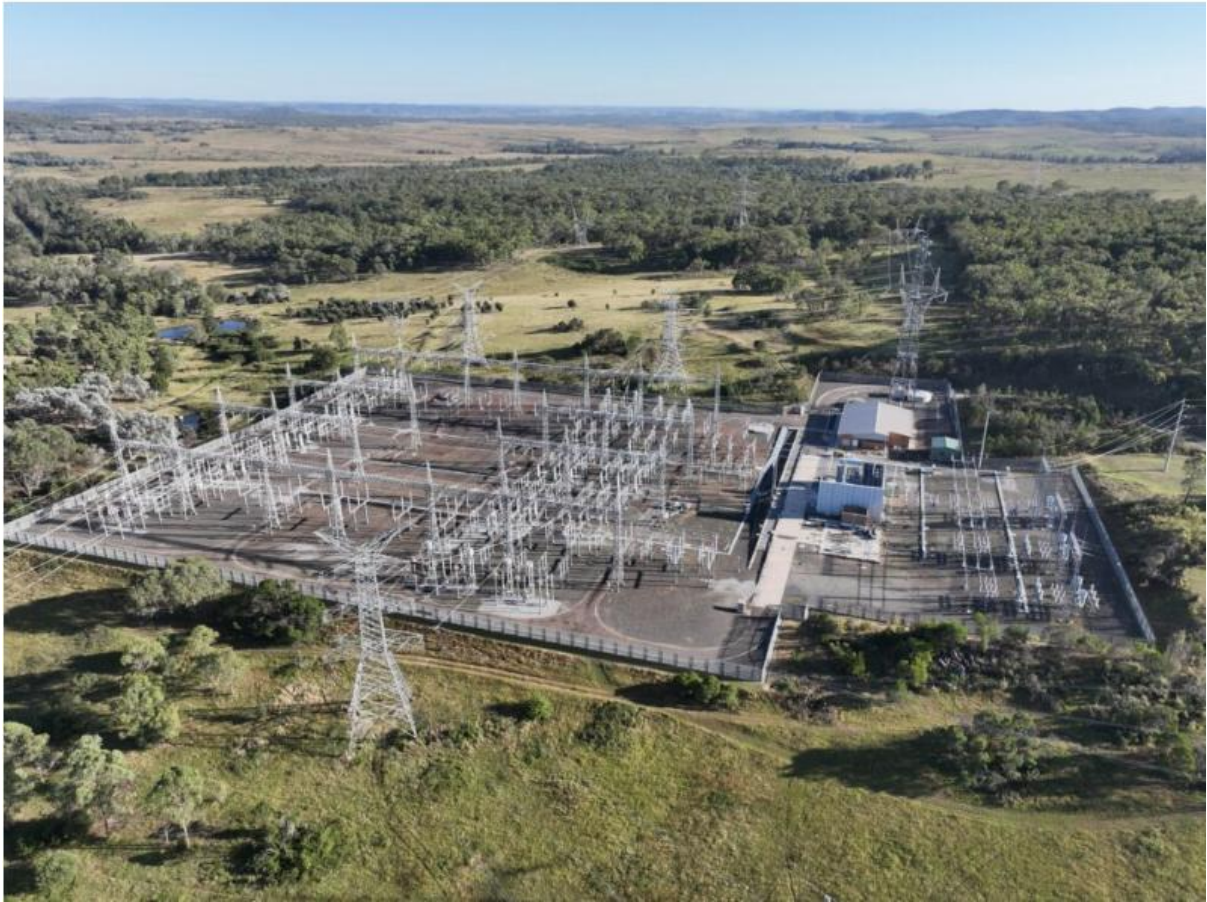
Figure 1: Existing Marulan Transgrid Substation
