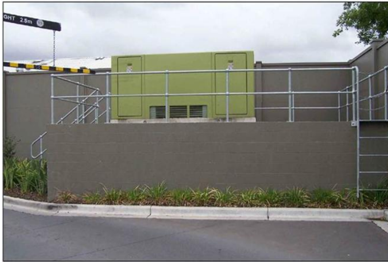
Figure 51 - Example substation raised above 1:100 flood level
