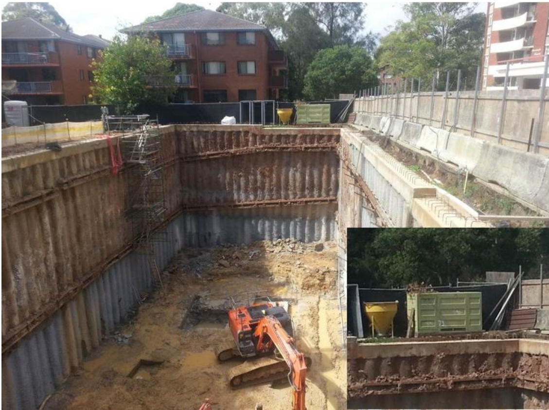
This excavation for a basement at 6 Sorrell Street Parramatta NSW for a mixed use 8 storey development in 2015 was identified by Endeavour Energy's Regional Services North as being unsafe due to the integrity of padmount substation 7858 located on the adjoining lot being compromised and access not being available. This resulted in the 'switching out' of the substation from the network until the site conditions were again deemed to be safe.
