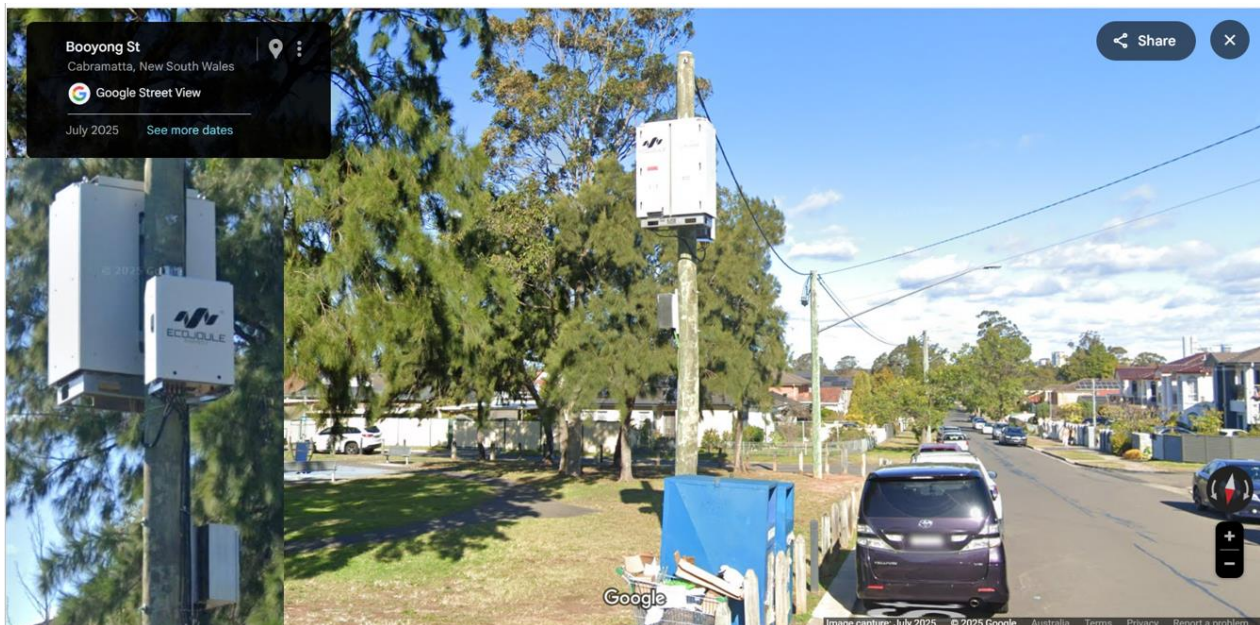
Battery unit, control box and distribution board on pole at Booyong Street, Cabramatta at Bolivia Park. Source: Google Maps Street View.
