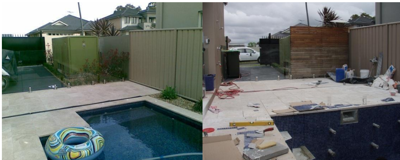
Before and After. This swimming pool in Endeavour Energy's network area at Middleton Grange NSW had to be modified to comply with the restriction for the padmount substation on the use of land in relation to swimming pools.
