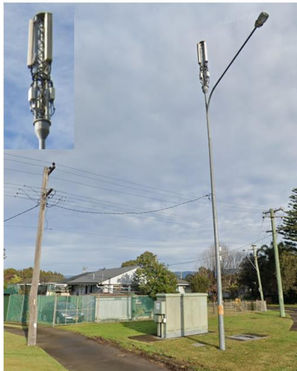
Telecommunications equipment on the road verge and streetlight column in Bedford Street and Northcliffe Drive, Berkeley. Source: Google Maps Street View.
