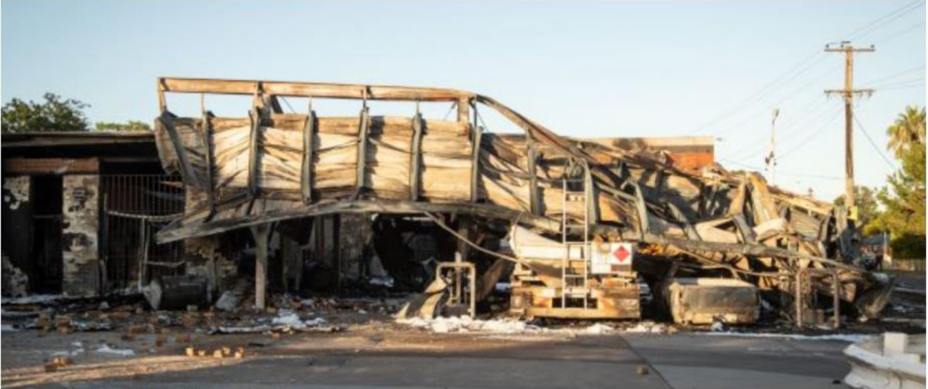
Figure 4: Service Station Facility Following Fire
