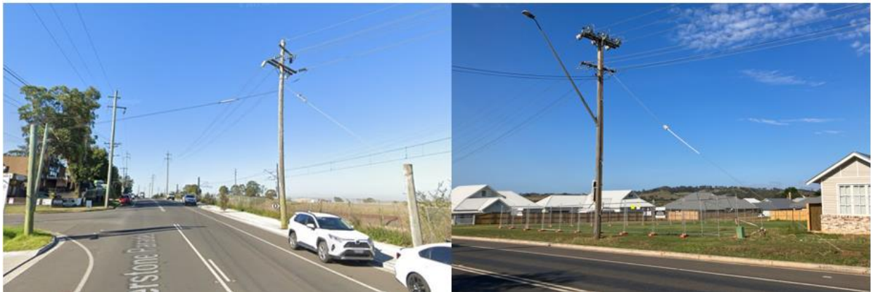
Stay poles at Riverstone Source: Google Maps Street View. Ground stay at Menangle which with the urban residential subdivision may need to be replaced with a bollard pole.
