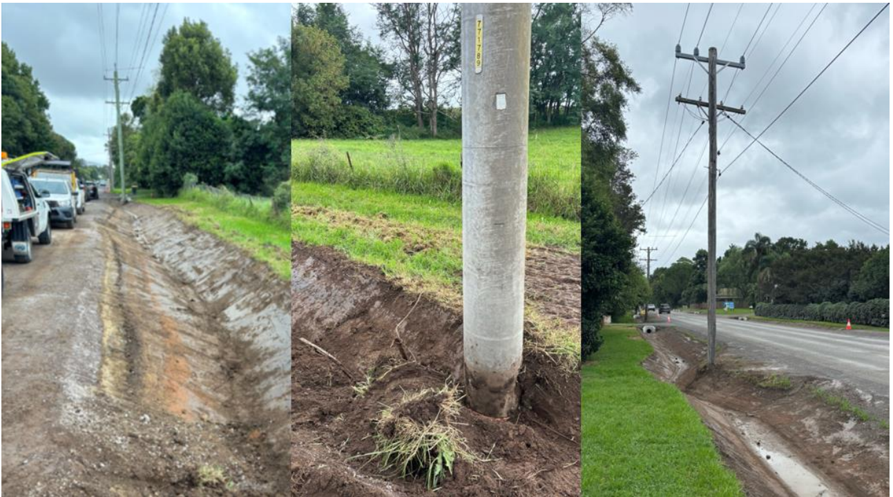
Crews from Endeavour Energy's Moss Vale Field Service Centre in March 2024 had to attend site as this excavation by a drainage contractor resulted in the striking of the earthing system for a pole mounted substation and compromised the support of the poles.
