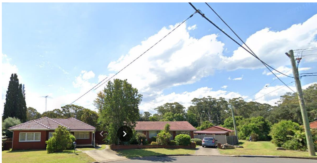
Mid span / suspended low voltage overhead service conductor for a dwelling at Rydalmere. Source: Google Maps Street View.
