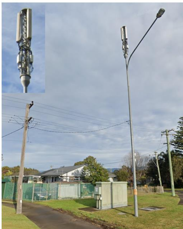
Telecommunications equipment on the road verge and streetlight column in Bedford Street and Northcliffe Drive, Berkeley. Source: Google Maps Street View.
