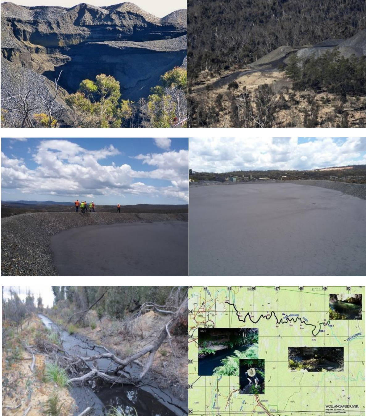
Photo 62-69: Clarence Colliery Reject Emplacement Area ("REA") 3 – collapsed on 2 July 2015
