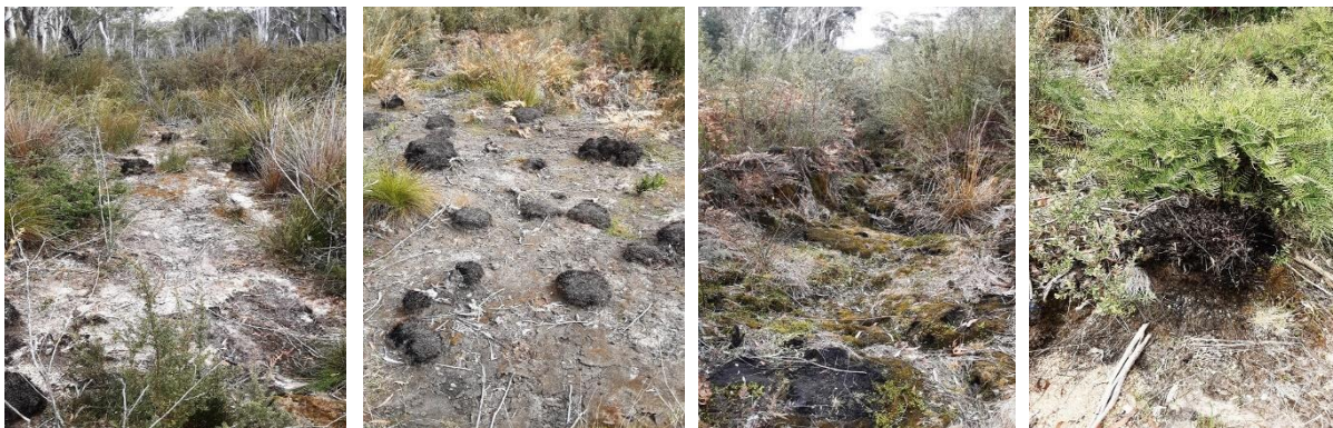
Photos 83-88: Site 22 – Banksia Swamp #2. Dry desiccated THPSS, erosion & nick points starting to occur.
