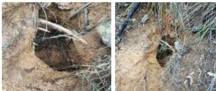
Photo 17 & 18: Site 6 Mine Subsidence Crack 600mm x 300mm – June 2024
