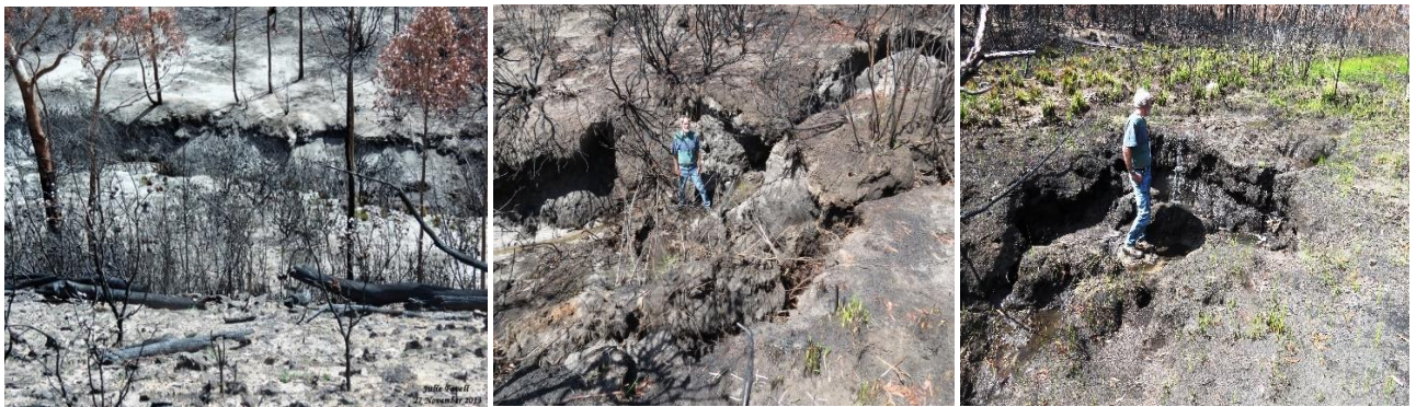
Photos 39, 40, 41: Site 12 – Erosion, scouring, slumping of THPSS in Farmers Creek swamp after 2013 Fire – 24 November 2013
