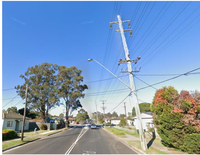
Overhead powerlines with high voltage, low voltage and service connections at different levels on the poles. This example is in Marayong NSW part of Endeavour Energy's franchise / network area. Source: Google Maps Street View.
