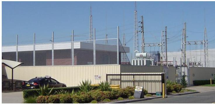
Endeavour Energy's Seven Hills Zone Substation is an 'outdoor' design. Note height of fencing due to adjacent 'climb point' created by the seating and awning. Source: Google Maps Street View.
