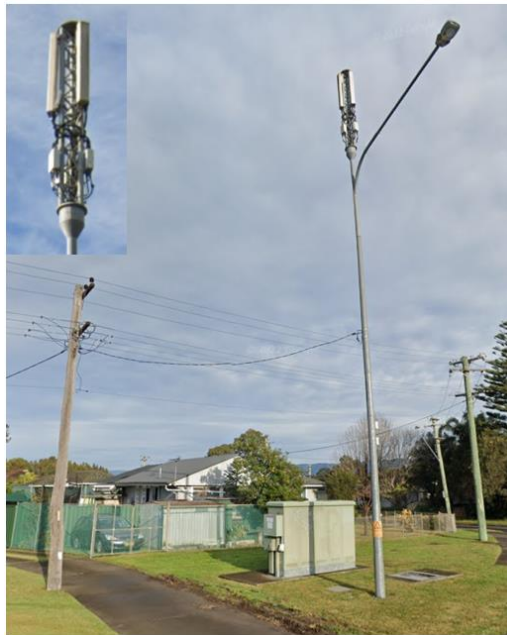
Telecommunications equipment on the road verge and streetlight column in Bedford Street and Northcliffe Drive, Berkeley. Source: Google Maps Street View.
