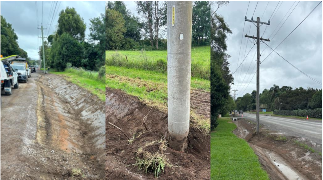
Crews from Endeavour Energy's Moss Vale Field Service Centre in March 2024 had to attend site as this excavation by a drainage contractor resulted in the striking of the earthing system for a pole mounted substation and compromised the support of the poles.
