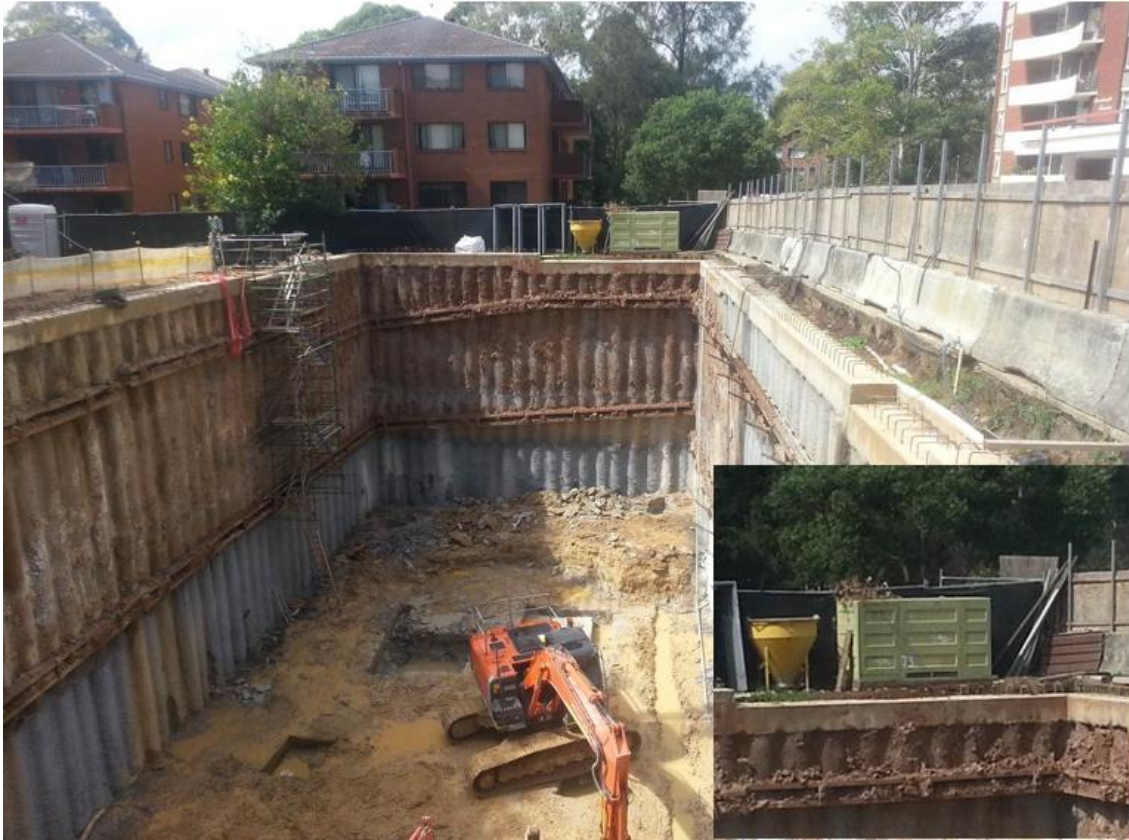
This excavation for a basement at 6 Sorrell Street Parramatta NSW for a mixed use 8 storey development in 2015 was identified by Endeavour Energy's Regional Services North as being unsafe due to the integrity of padmount substation 7858 located on the adjoining lot being compromised and access not being available. This resulted in the 'switching out' of the substation from the network until the site conditions were again deemed to be safe.
