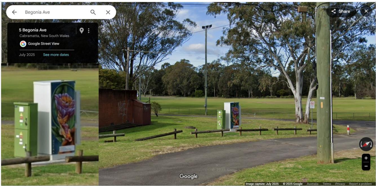
Battery unit and distribution board installation at Begonia Avenue, Cabramatta at the entrance to Don Dawson Oval (Cabramatta Sports ground). Source: Google Maps Street View.
