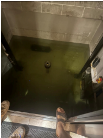
Flooded lift well at apartment block on Wilberforce Avenue Rose Bay. Owners have been advised to hire a water engineer to address groundwater penetration issues that have likely been caused by settlement from recent two level basement excavations on Old South Head Road in Rose Bay..
