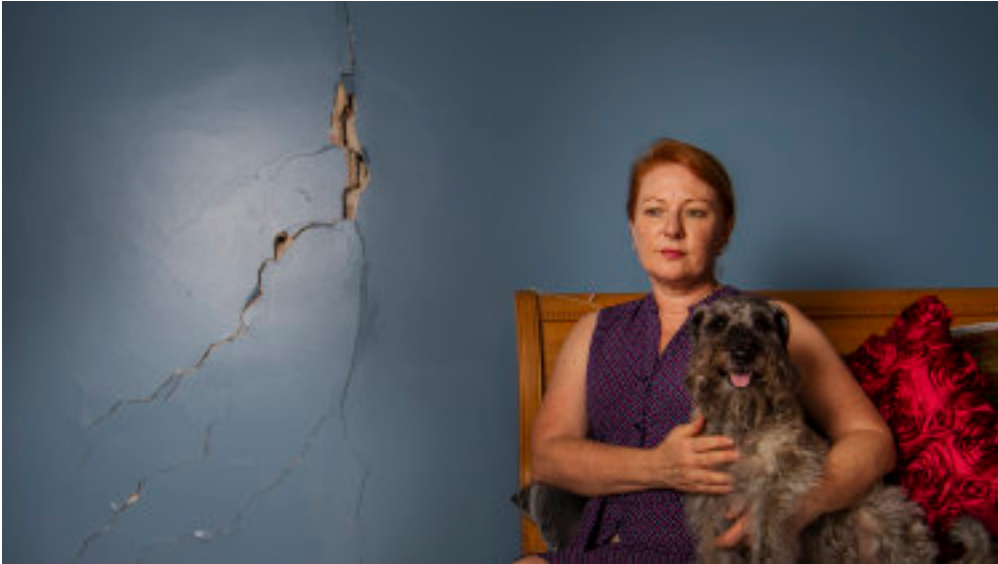
3. CARRINGTON ST STRATHFIELD DAMAGE –CAUSED BY TUNNELLING 40MTRES BELOW
