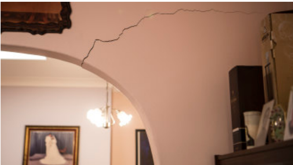
4. CARRINGTON ST STRATHFIELD DAMAGE CAUSED BY TUNNELLING 40MTRES BELOW
