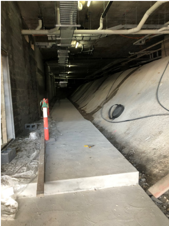
Figure 5: Showing water storage area
