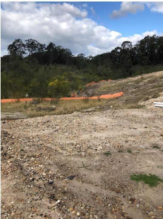
Figure 3: Showing Sediment controls at boundary
