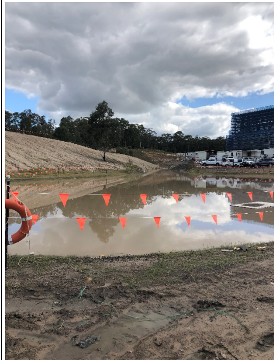
Figure 4: Showing sediment basin at capacity after heavy rainfall
