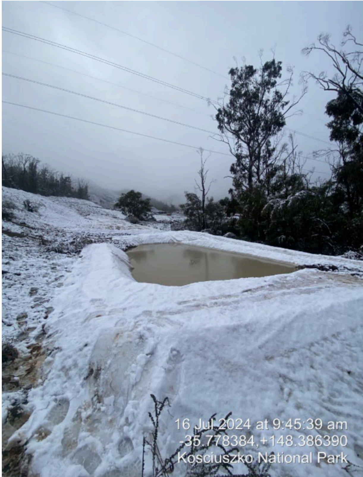
Figure 7: Sump A during rainfall after rectification works. No signs of leakages were identified during the inspection.
