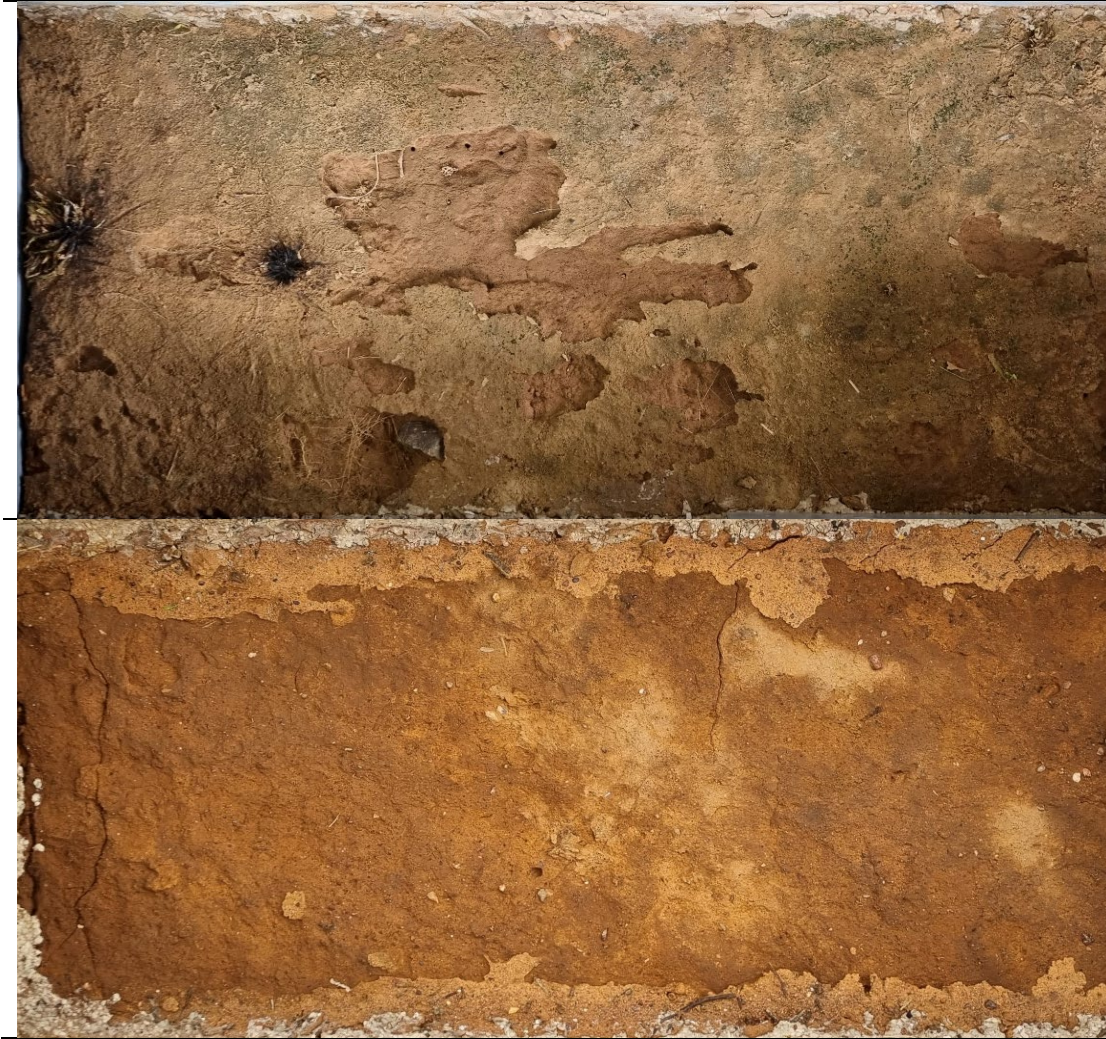
Figure 16: Examples of scoured surfaces generated by application of overland flows.
