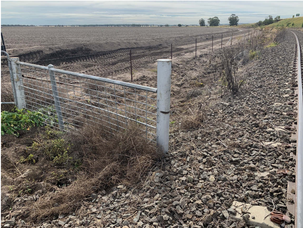
Appendix 3: View of the fencing of the pen leading into the Newell Highway underpass at the crossing of the existing shunt rail line. Currently low points such as this provide escape opportunity for moving stock. (Orientation: North)
