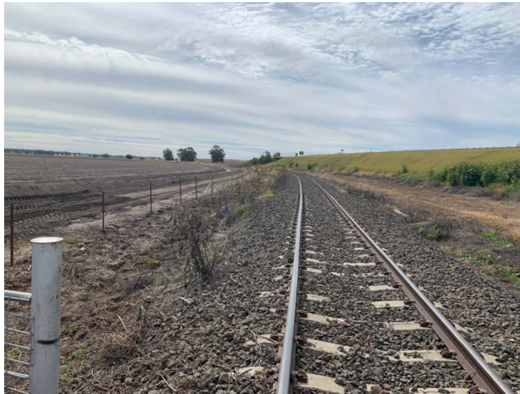
Figure 1-4: Shunt rail line on western exit of existing under pass (Orientation: North)
