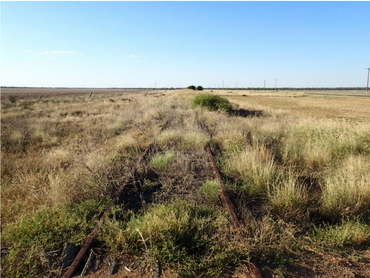
PHOTOGRAPH 3.2 INDICATIVE CONDITION OF EXISTING TRACK WITHIN THE BOGGABILLA RAIL CORRIDOR (DATED 10 APRIL 2018)
