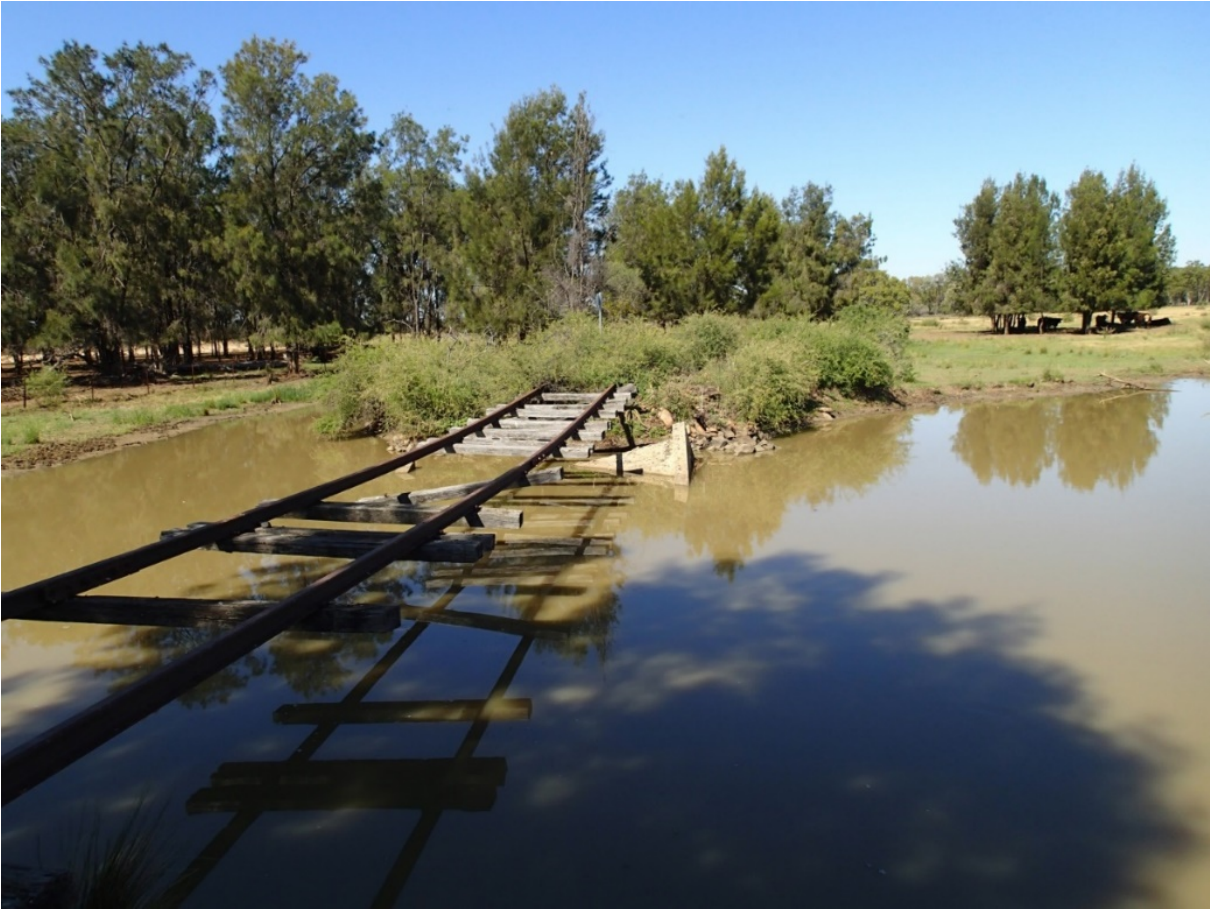
PHOTOGRAPH 3.1 DERELICT TRACK WITHIN THE BOGGABILLA RAIL CORRIDOR (DATED 9 APRIL 2018)
