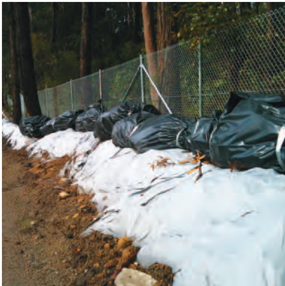
FIGURE 7.11: Removed vegetation was securely wrapped in black plastic bags before disposal to prevent the spread of the pathogen Myrtle rust on the M2 Upgrade, Sydney region (Photo: Nicholas Francesconi).
