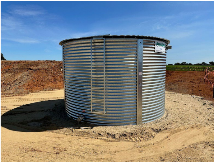
Photo 17: 20kl Water tank (Camp 2)
