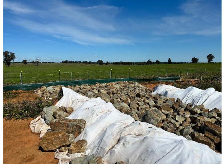
Photo 18: Sediment basin outlet with geofabric and rock scour protection
