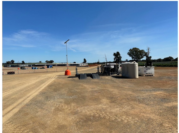
Photo 16: Wheel wash facility – Camp 2
