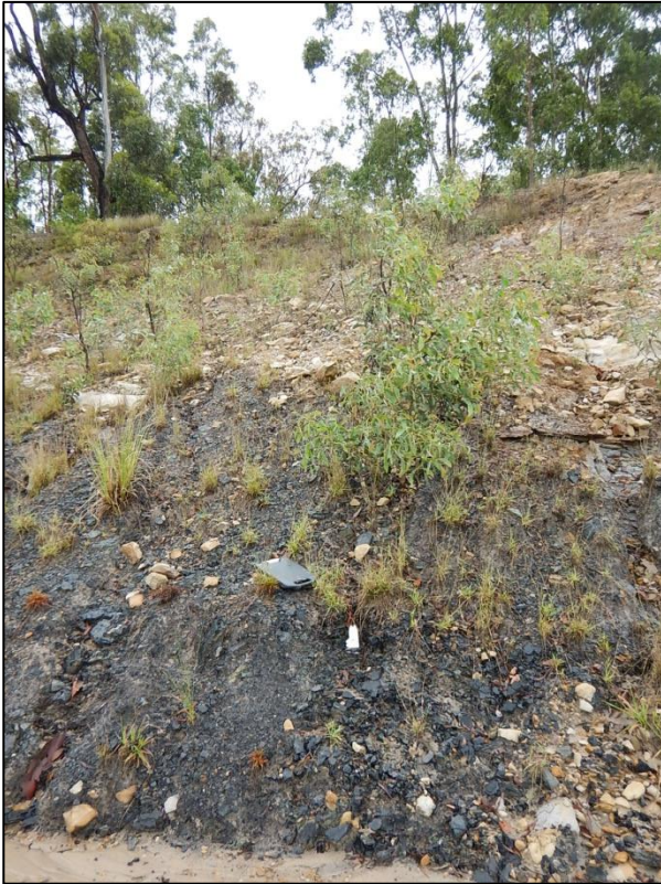
Figure 20: Coal exposed in lower area of batter
