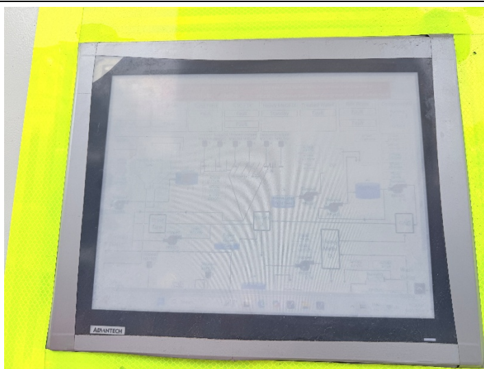
Photo 34: Site Compound C3 - The water treatment plant control panel allows operators to monitor the treatment process, including in-line parameters such as inflow and discharge turbidity and pH.
