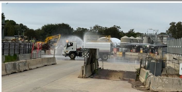
Photo 22: Site compound C1 – Operational water cart was observed on multiple occasions during the site inspection at various locations.
