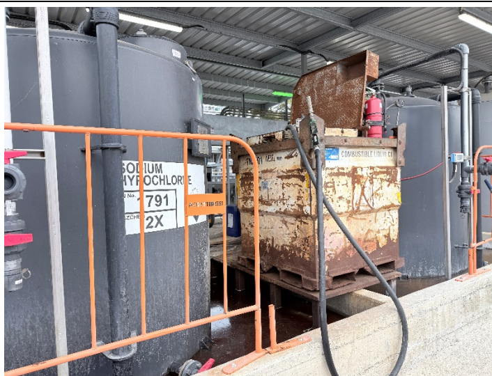
Photo 35: Site Compound C3 – Diesel fuel tank located under cover and within secondary containment. The bund contained accumulated rainwater and required cleaning out.
