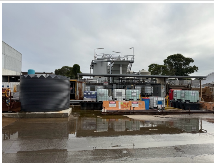
Photo 28: Site compound C2 water treatment plant as per EPA EPL No. 21600
