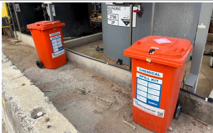
Photo 25: Site compound C1 – Adequately stocked chemical spill response kits observed at various locations across the compound, including immediately adjacent to the water treatment plant.
