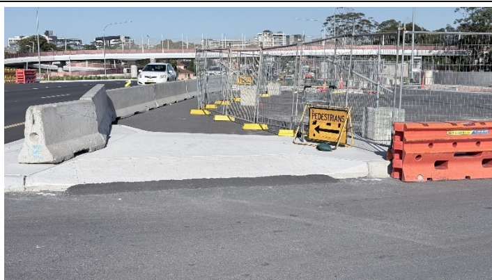
Photo 16: Presidents Ave - Pedestrian wayfinding signage installed on President Avenue adjacent to the M6 tunnel portals.
