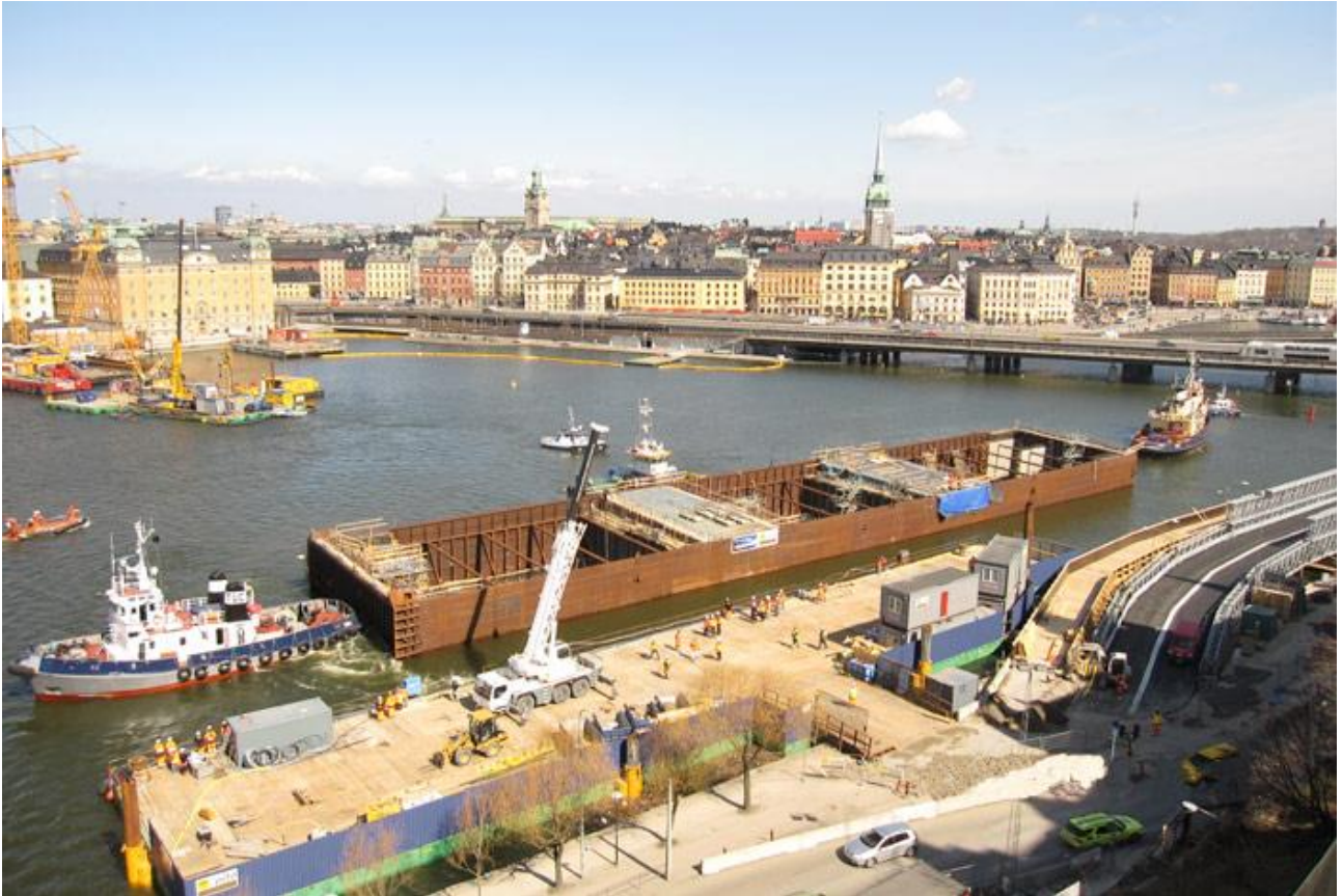
Figure 6-16 Example of a casting facility for the Soderstrom Tunnel, Stockholm (Source: TunnelTalk, 2013)
