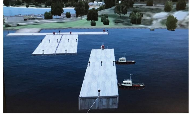
Steel shell unit arrives at Spit West Reserve construction support site (BL9) casting facility.
