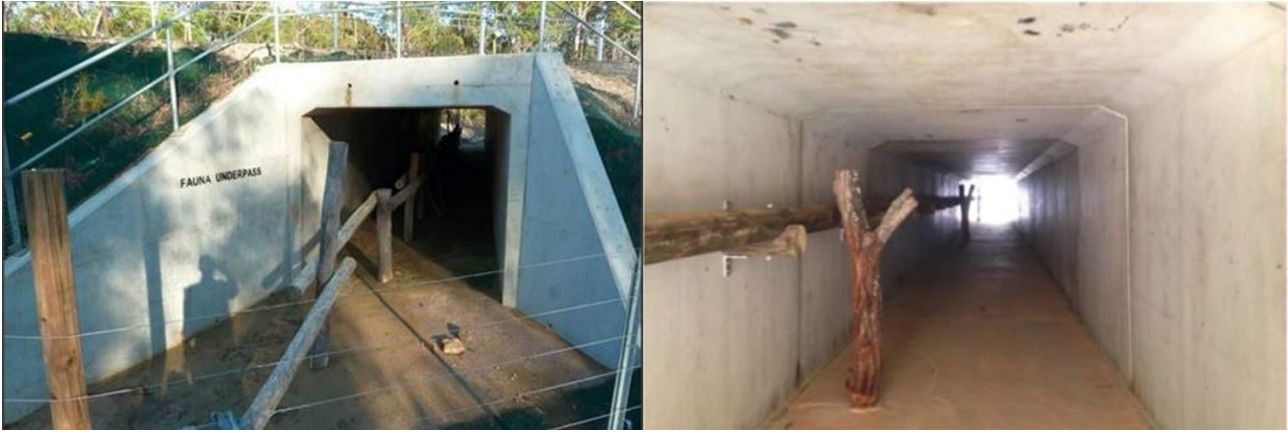
Figure 6-22 Example of a fauna underpass (Pacific Highway Upgrade, Woolgoolga to Ballina upgrade)
