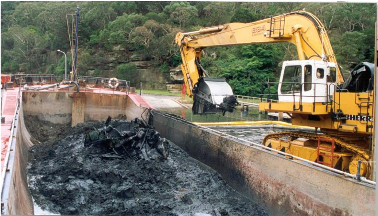
Figure 6-14 Example of an excavator fitted with a closed environmental clamshell loading into a hopper barge (Source: supplied by Royal Haskoning DHV, 2020)
