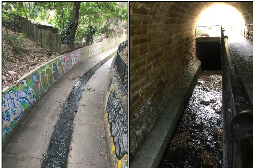
Figure 3-3 Flat Rock Creek at the upstream site looking upstream (5a) (left) and along the underground channel (right)
