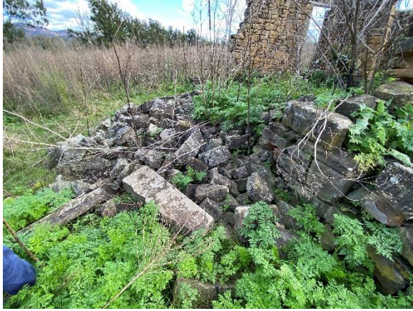
Figure 4-17: View of the collapsed easterly wall.
