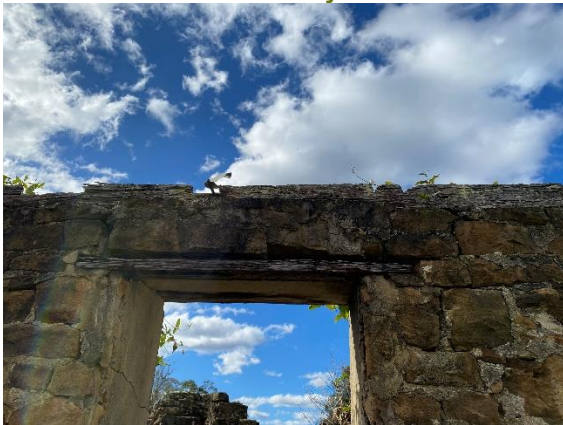
Figure 4-27: Example of timber lintel and timber framing to former roof with evidence of metal bracket nailed to the beam.
