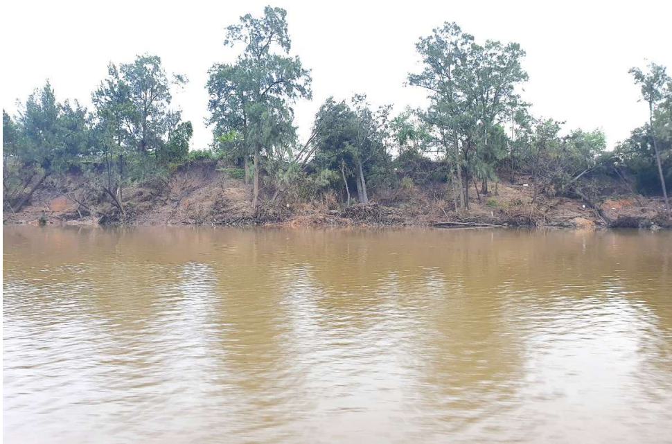
Image 6. Riverbank in the Wilberforce area. Note significant erosion from recent flood events with significant undermining of the riparian vegetation.
