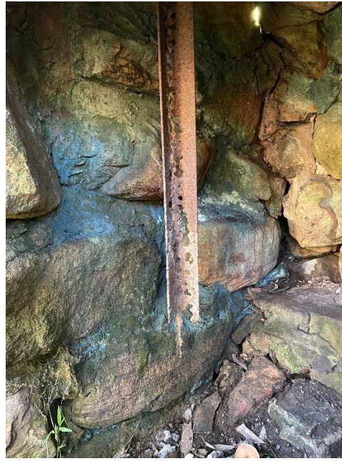
Figure 4-14: Closer image of the iron bar vertically hanging within the fireplace.
