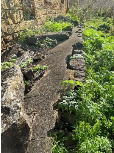
Figure 4-19: View of the subsided veranda.
