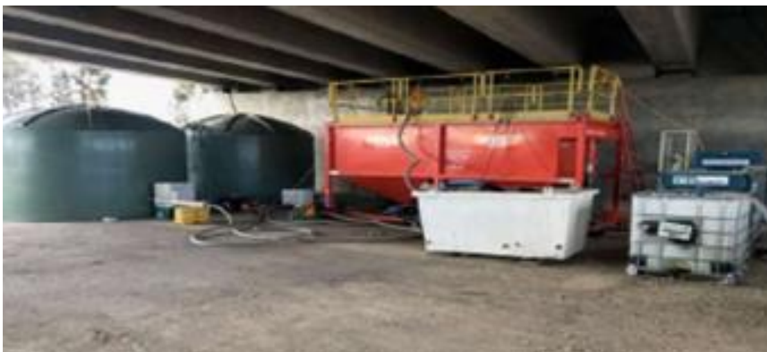
Photo 1 Example of water collection, treatment and reuse plant
