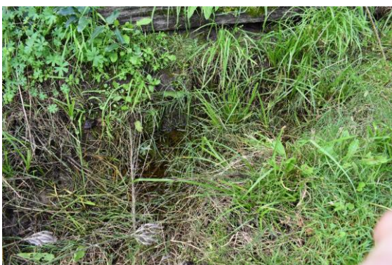
Figure 4-39: Example of damp ground beneath the foundations.
