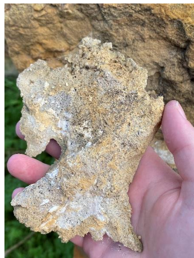
Figure 4-34: Flaked lime wash from the walls, showing sand aggregate.
