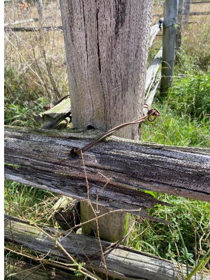
Figure 4-47: Example of the high tensile fencing wire used to tie the rails to the posts at the yard.
