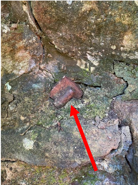
Figure 4-11: Image of one of the steel bolts protruding from the side of the chimney.
