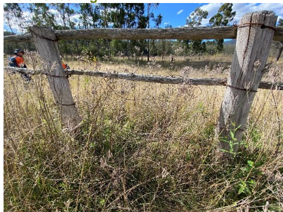
Figure 4-51: Another example of the condition of the timber fencing at the yard.
