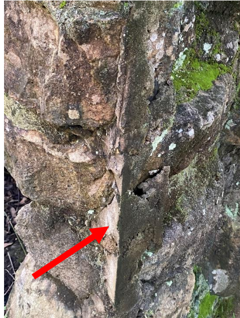
Figure 4-12: Image of one of the external sides of the chimney, showing possible former joint or wall.
