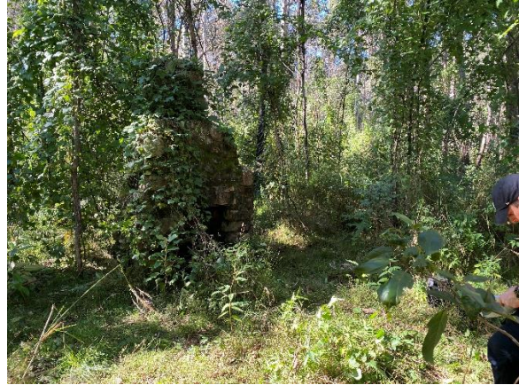
Figure 4-8: View of the chimney showing vegetation growing over the structure.
