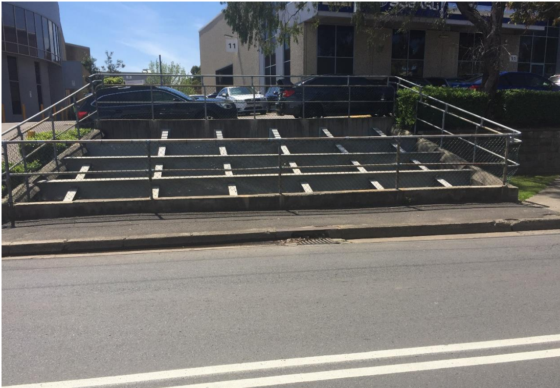
Figure 16 Considerable stormwater structure at Clay Cliff Creek, River Road West (Source - Arup)
