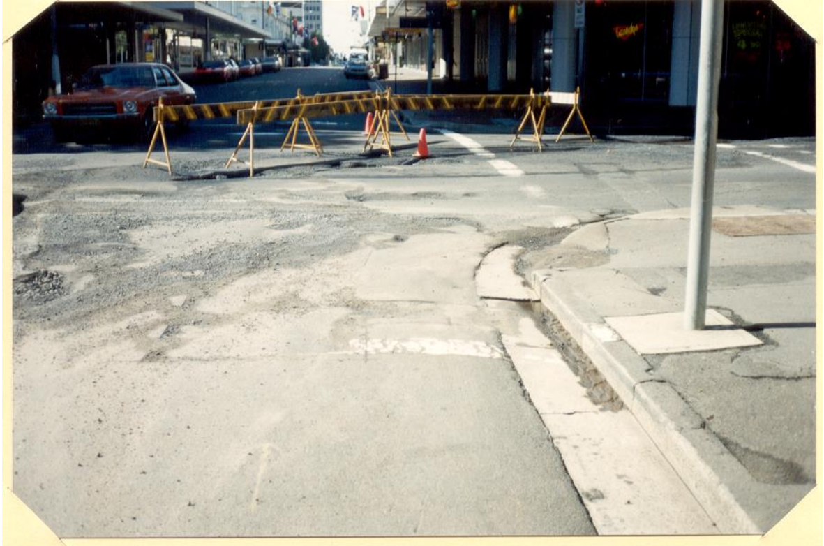
Figure 15 Scouring of asphalt at Marsden Street / Macquarie Street due to overland flow, 30 April 1988 (Source - CoP)
