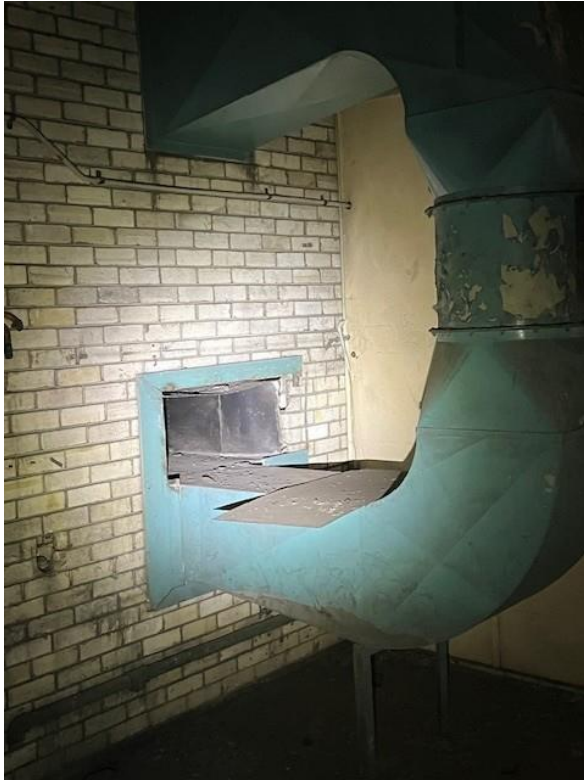
Photograph 19: Ventilation duct within dark room
