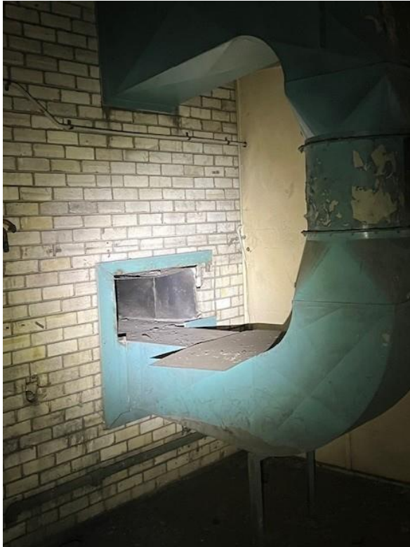
Photograph 19: Ventilation duct within dark room
