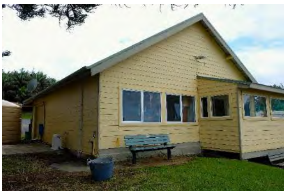
PHOTOGRAPH 4-34 CARGO SHED WEST ELEVATION WITH 1980S ADDITION TO BE REPLACED WITH DECKING
