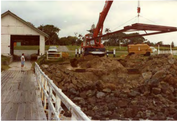
PHOTOGRAPH 4-18 WORKS DURING INITIAL STAGES OF CONSTRUCTION OF NEW JETTY, GABLE END IS STILL CLAD WITH FIBROUS CEMENT SHEETING WITH TIMBER BATTENS. C.1982 (LHI MUSEUM)
