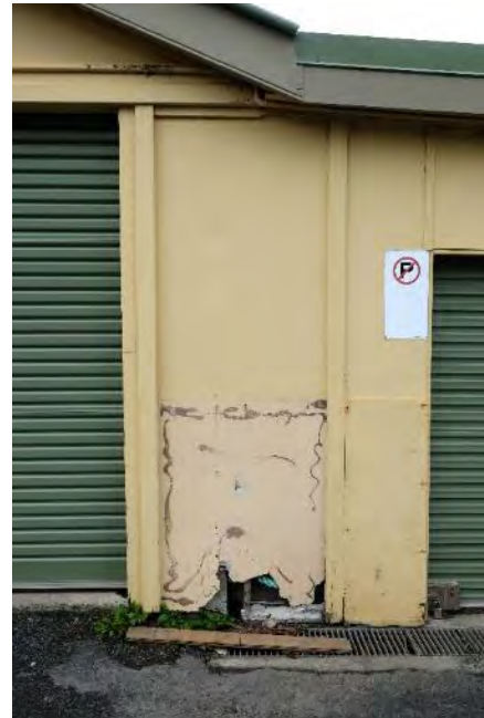
PHOTOGRAPH 4-41 PANEL DAMAGE TO EAST ELEVATION
