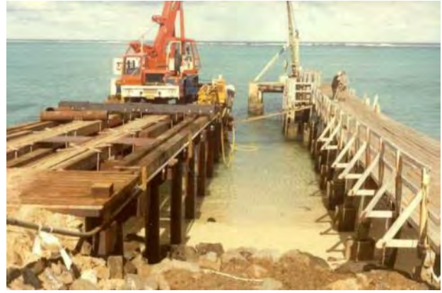
PHOTOGRAPH 4-19 CONSTRUCTION OF THE NEW JETTY, 1982. OLD JETTY (AT RIGHT) WAS CONSTRUCTED IN 1956 (LHI MUSEUM)
