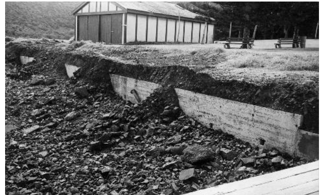
PHOTOGRAPH 4-17 STORM DAMAGE TO RETAINING WALL, OV SHED IN BACKGROUND, C.LATE 1960S/EARLY 1970S (LHI MUSEUM)
