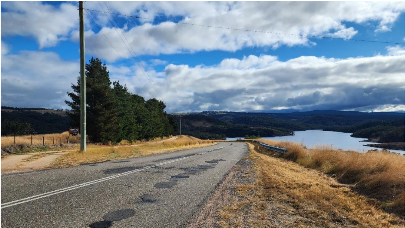
Photograph 3.1 Potholes along Magpie Hollow Road (view from east towards Lockyers Line)
