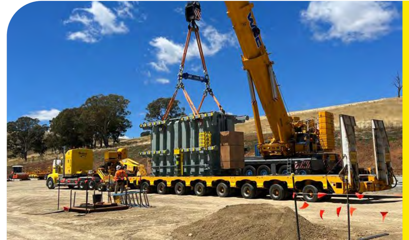
Above: ARES delivering 125T power transformer (without oil) to Flyers Creek Wind Farm on BR8 Platform trailer.
