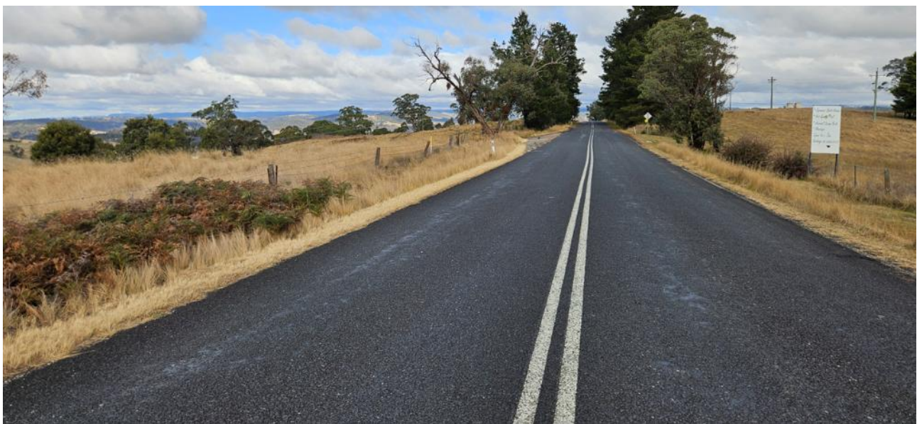
Photograph 3.4 Rural section of Magpie Hollow Road (view from Sir Thomas Mitchell Drive)
