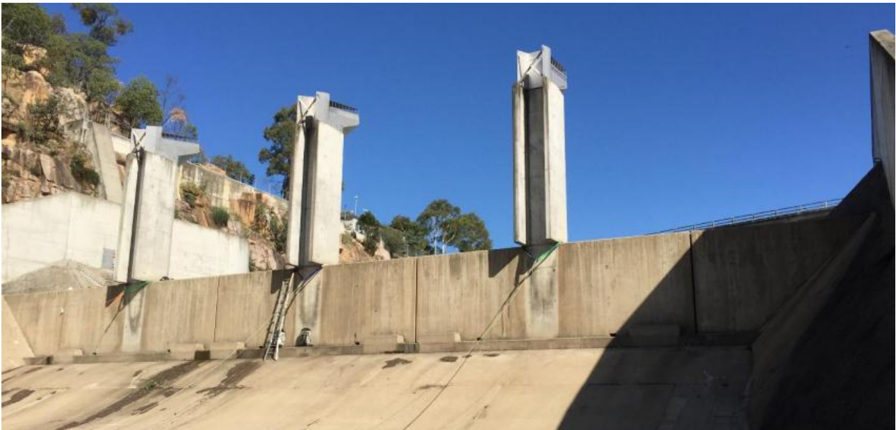
Figure 4.10 Lake Lyell hydroplus fusegates - view from downstream
