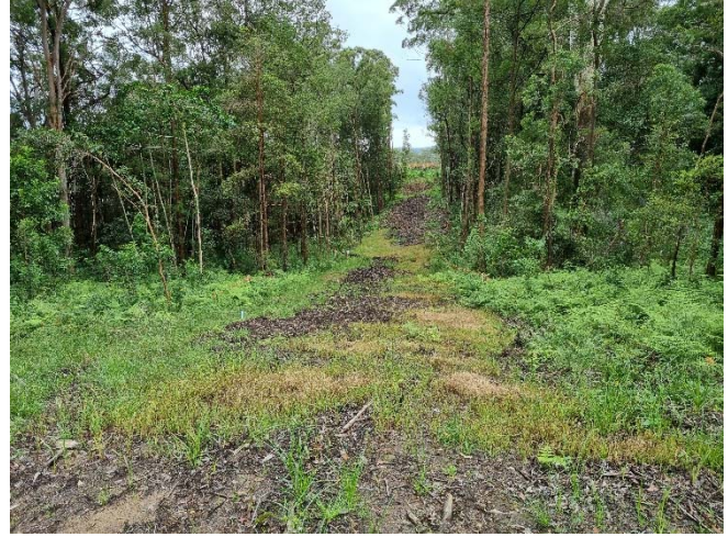
Image 2: Stabilisation and revegetation of clearing corridor (Ch 10200 to 10400, west side of highway)
