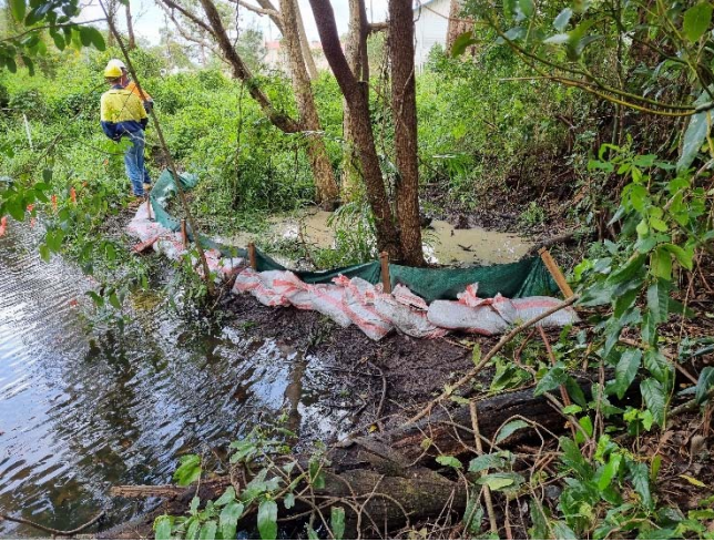
Image 1: Isolated turbid water generated by HDD frac-out environmental event (15/03/22)
