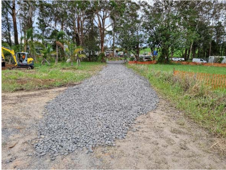
Image 5: Englands Rd Dewatering Area – site access and flagged off aboriginal heritage salvage area on right
