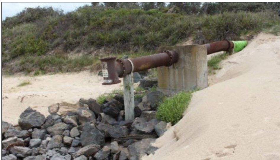
Figure 1-1: Current beach-face outfall pipeline
