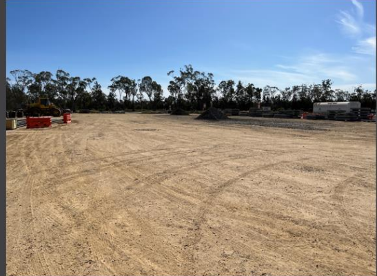
Pad 6 adjacent to occupied house site of dust generation by travelling vehicles. Dust control required
