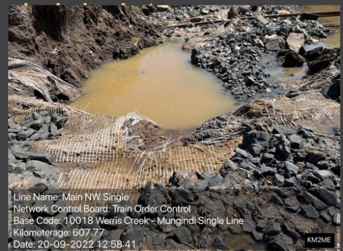
Downstream damage at Boggy Creek requires stabilisation
