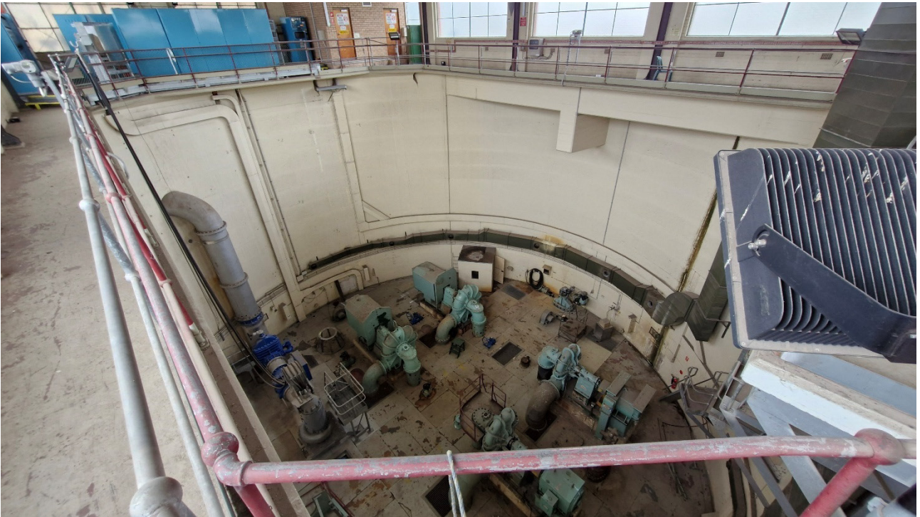
Plate 6.18 View of internal substructure including circular concrete structure and 1960s pumping units
