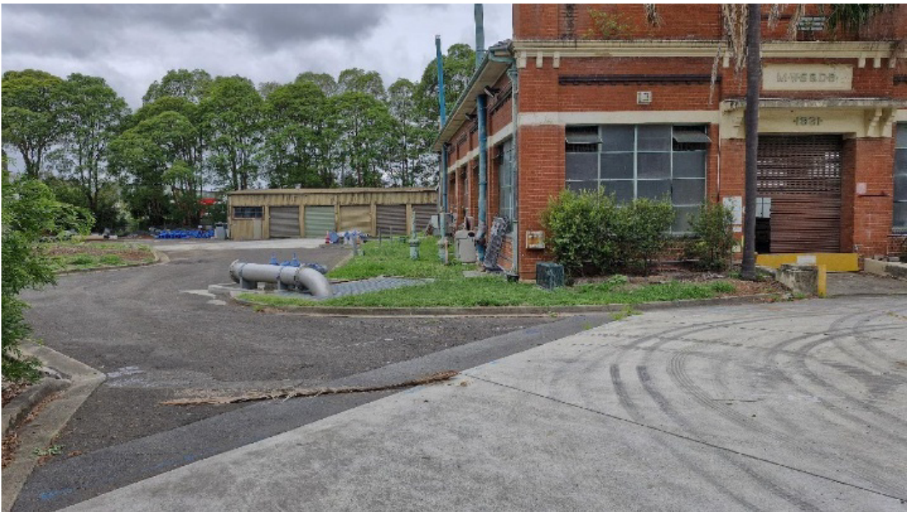
Plate 6.10 Sewage Pumping Station 067 structure on the right, with the pipeline alignment on the left. View east.
