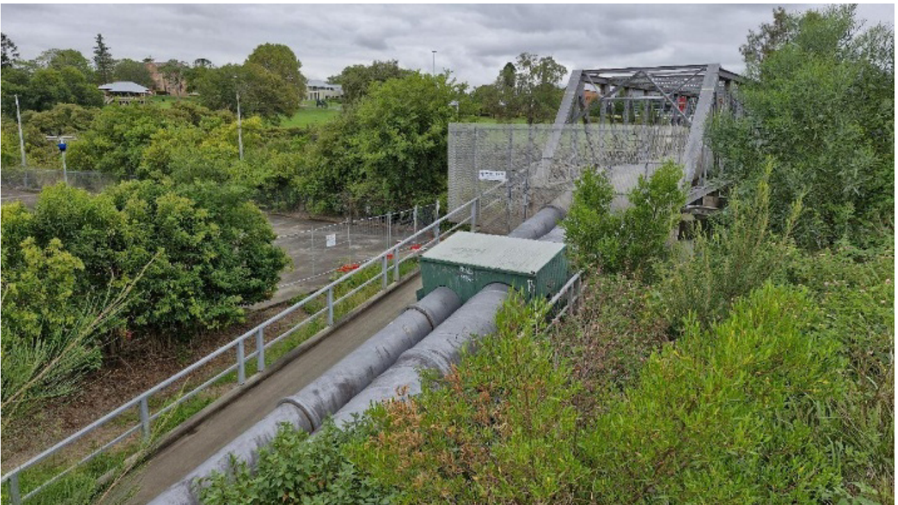
Plate 6.9 Sydney Water pipe infrastructure River crossing. View north-west.
