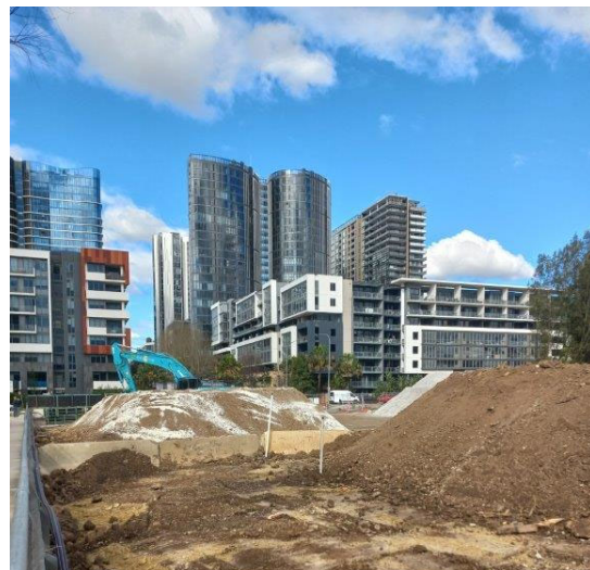
Photo 24 View east across former substation off Hill Road, stockpiles and monitoring wells present across this site.
