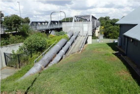
Plate 19. View to south-west. Parramatta campus of Western Sydney University. Existing water pipelines on northern side of the Parramatta River. Highly disturbed ground.
