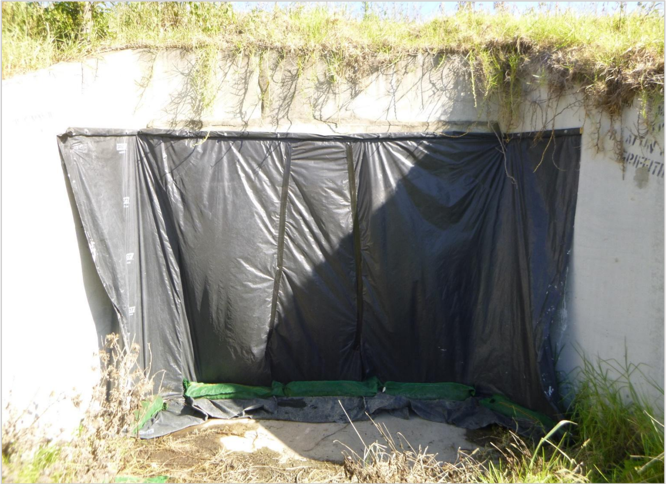
Figure 6-1 An example of 'Bat Curtains' used to exclude a culvert from Microbat entry
