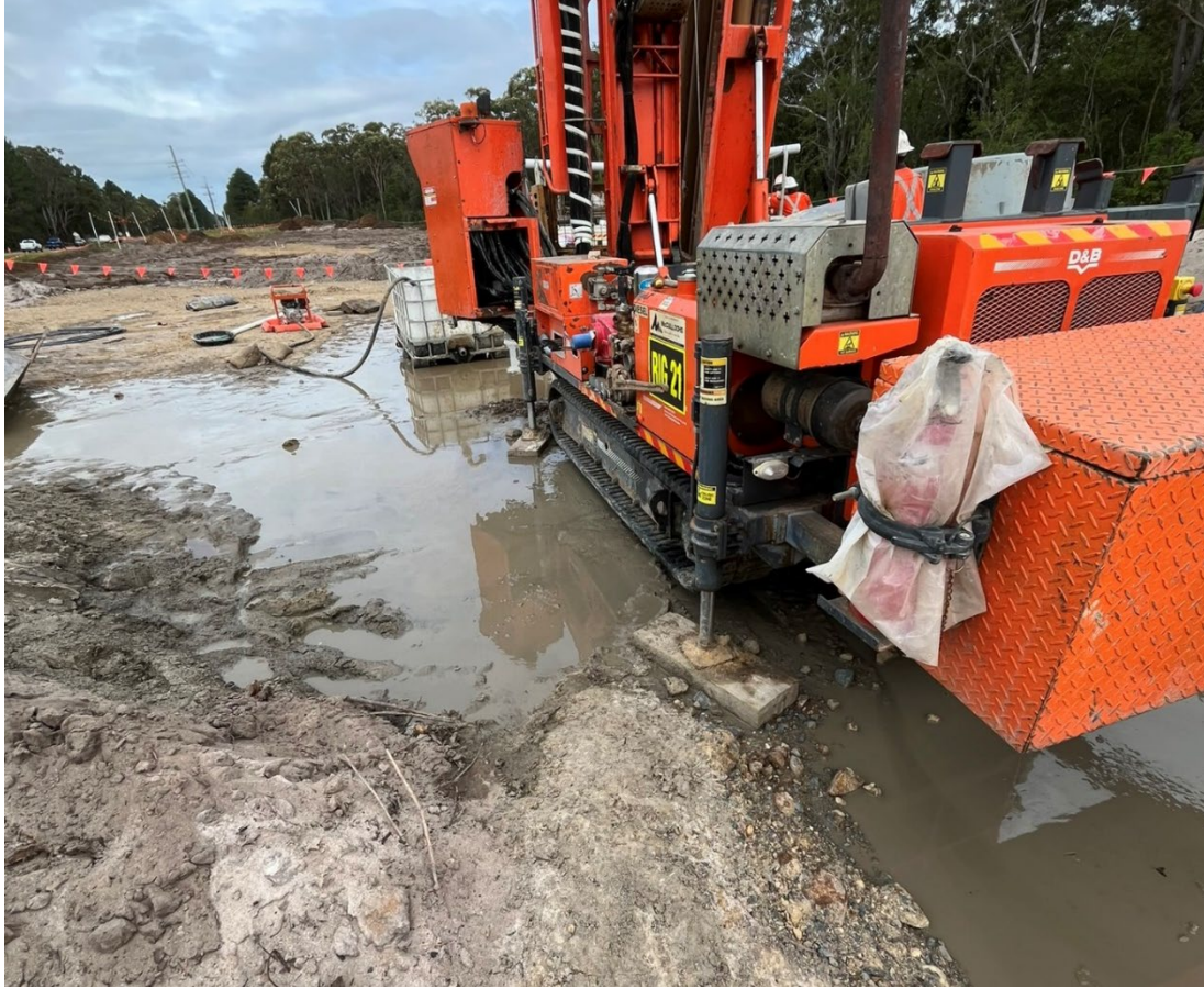
Photo 16: Uncontrolled waste water from drilling operations near Gate 4, HB 4B
