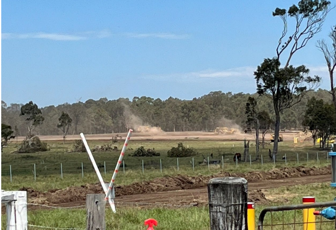
Photo 3: Excessive dust generation from scraper operations at AS3 – BH2T
