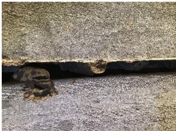
Photograph 41: Shallow gaps where culvert sections are joined may provide roosting opportunities
