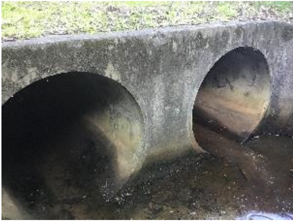
Photograph 38: Double 1050 mm culvert under Old Punt Road provides the best roosting opportunities
