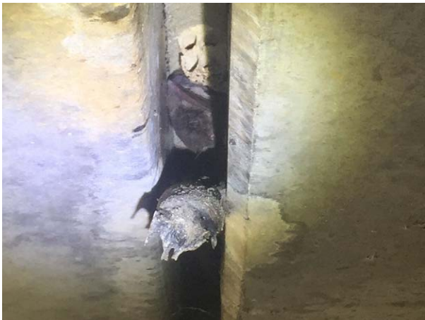
Photograph 36: A single Little Bent-winged Bat ( Miniopterus australis ) roosting under the Pacific Highway bridge over Windeyers Creek
