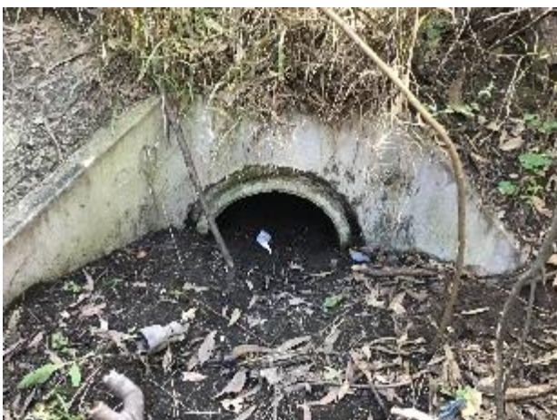
Photograph 42: 500 mm culvert on Lenaghans Drive half filled with sediment
