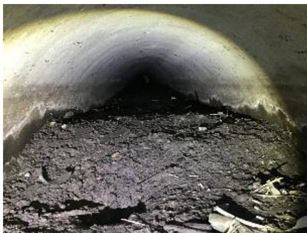
Photograph 43: The view inside a 500 mm culvert on Lenaghans Drive filled with sediment
