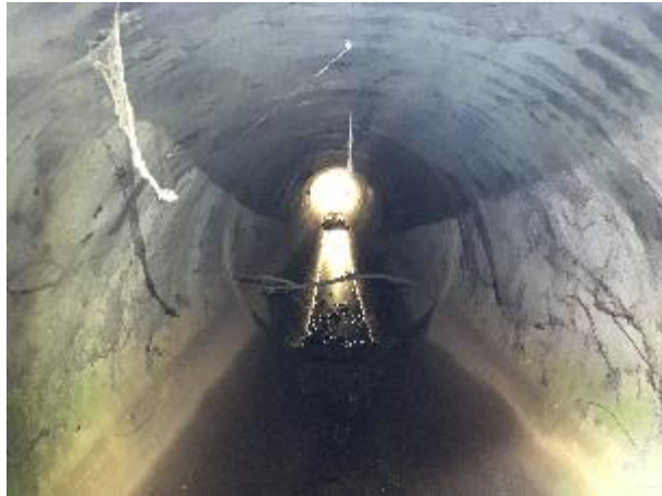
Photograph 39: The view inside a 1050 mm culvert under Old Punt Road shows an abundance of cobwebs suggesting no recent use
