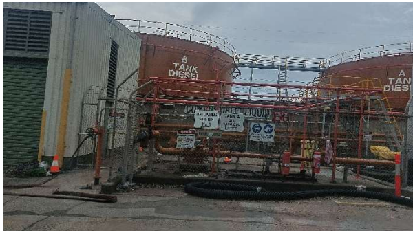
Photo 6. Fuel tank farm – multiple diesel and water tanks and supporting infrastructure
