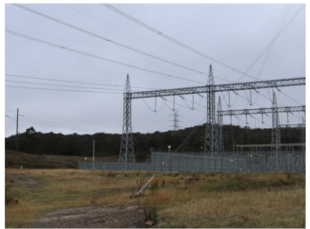
Mount Piper 330 kV Substation
